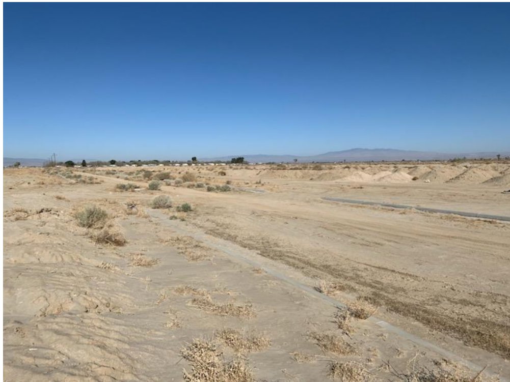
24. View northeast from northeast portion of property. Showing limited curb and gutter installation.
