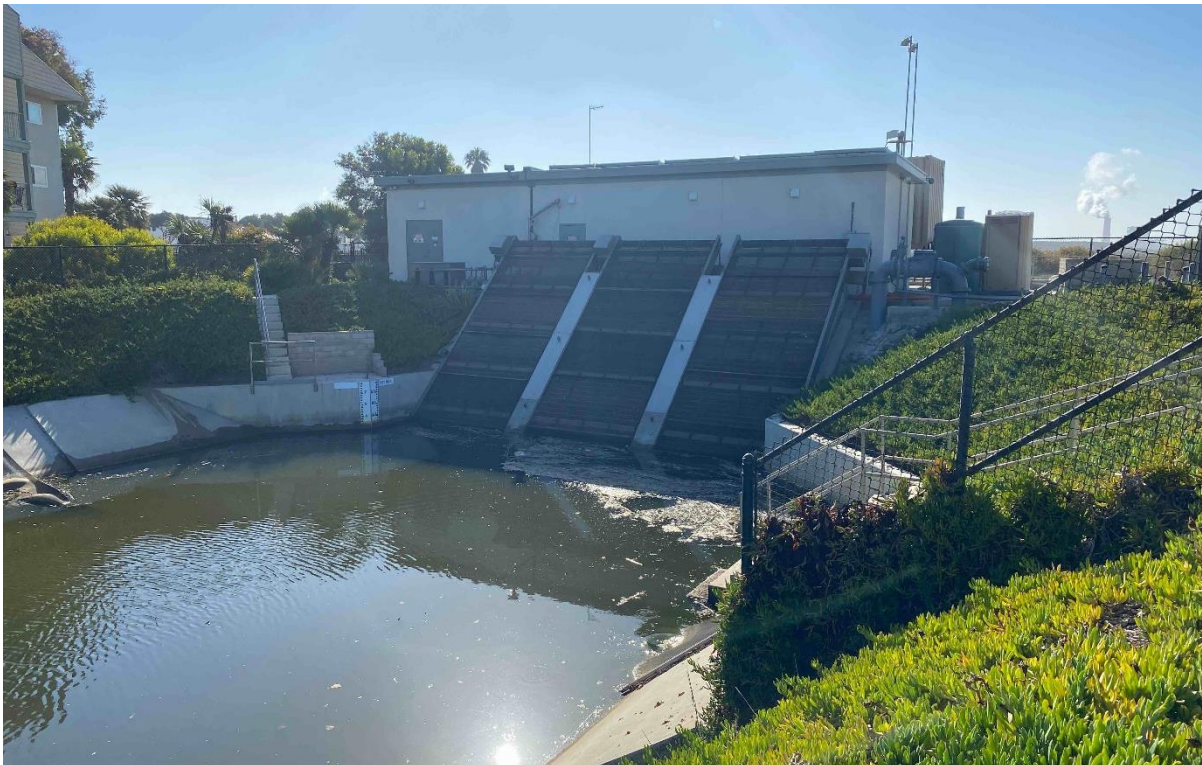
Photograph 2. View of J Street Pump Station at the southern end of Bubbling Springs. Aspect: east. Date: 8/4/21.
