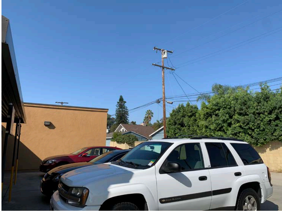
Photo 9 – Pole-mounted electrical transformer located along the alleyway to the north.
