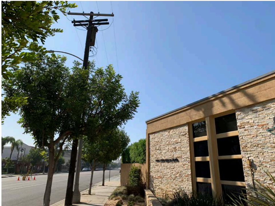
Photo 8 – Encased pole-mounted electrical transformer located along Long Beach Boulevard – adjacent to the east of the Property.
