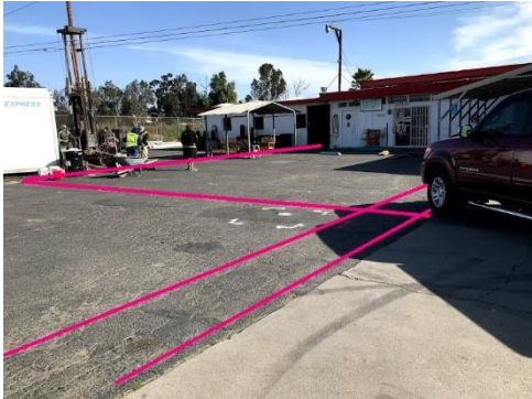
Photo showing where unknown piping was located either with an EM pipe locator or GPR.
