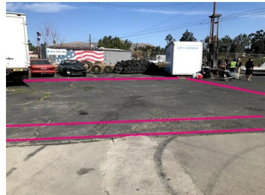
Photo showing where unknown piping was located either with an EM pipe locator or GPR.
