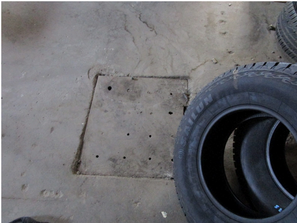
18. Drain cover inside lift area in 13906
