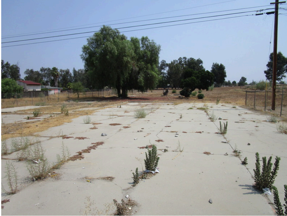
5. Foundation remnants at 13856 Old Frontage Road, northwest side of the subject property
