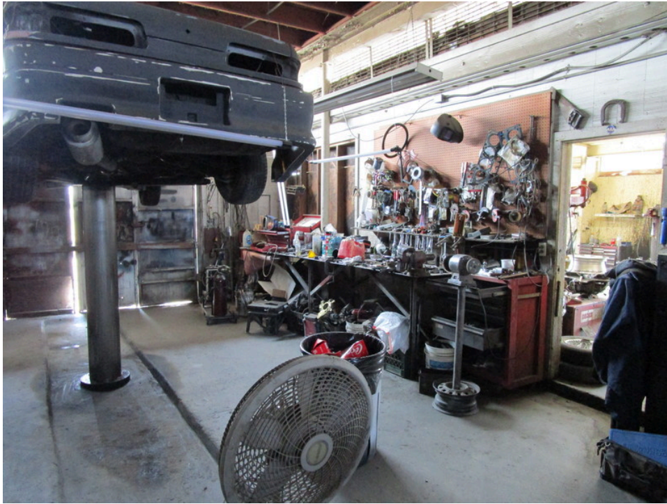
17. Hydraulic lift inside P&B Tires on subject property
