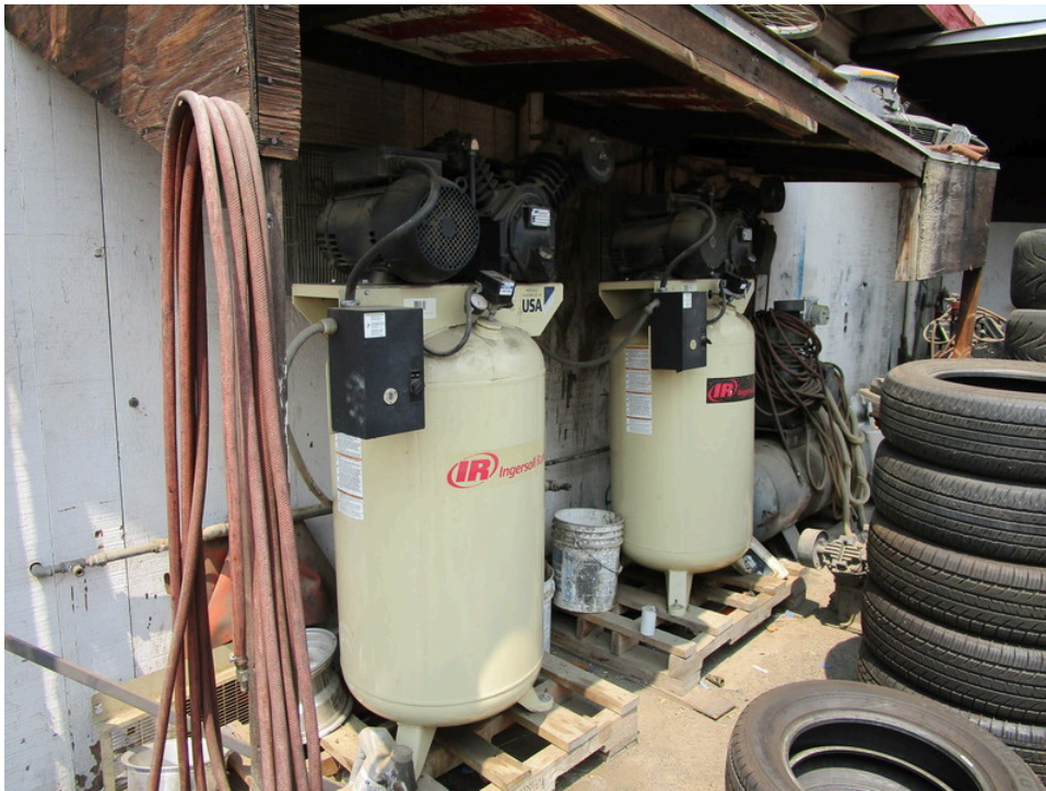
16. Air compressors at subject property 13906
