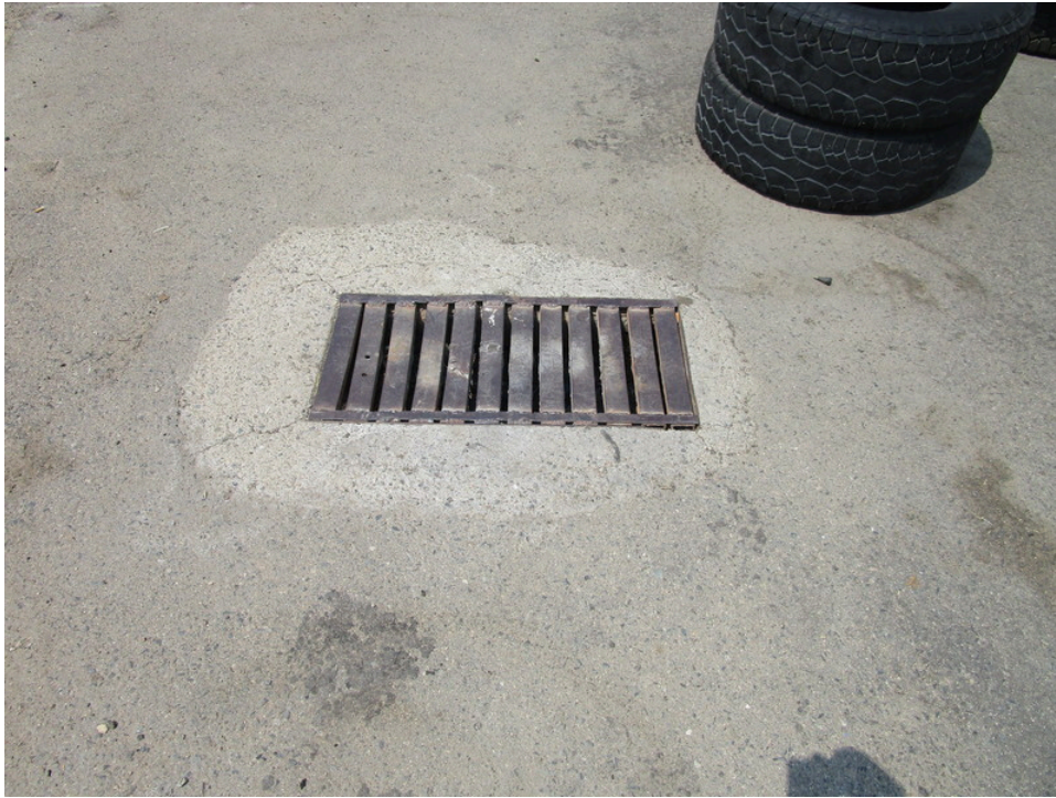
15. Drain on subject property 13906
