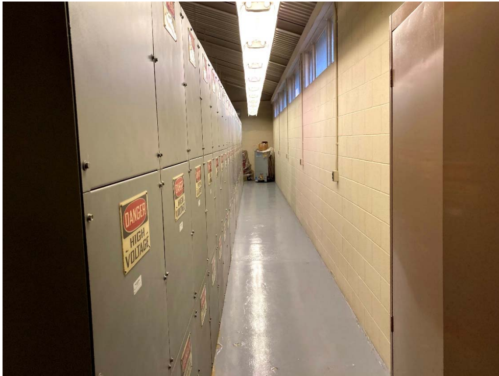
Photo 4: The view is from the northwestern corner of the control room to the south.
