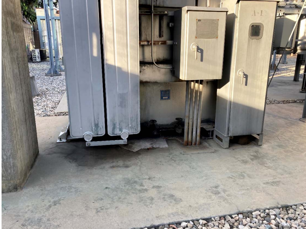
Photo 13: A small transformer oil leak was present below the southernmost transformer. The leak was old, controlled with absorbent, and did not extend beyond the concrete pad.
