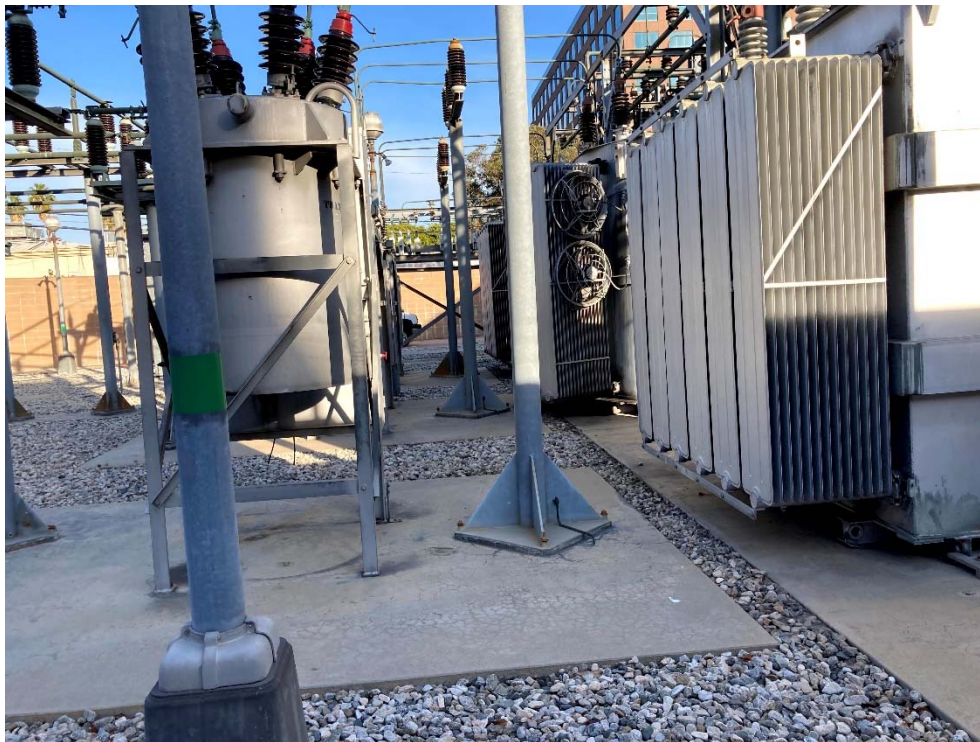
Photo 14: The reverse side of the transformer with the small leak is at photo right. The view is to the north.
