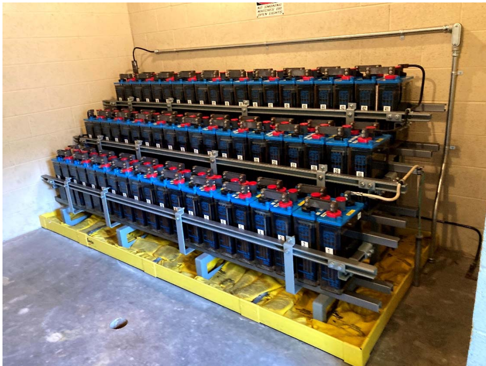
Photo 6: The bank of lead-acid batteries at the southern end of the control house was in secondary containment. A small bathroom was located between the control room and the battery room.
