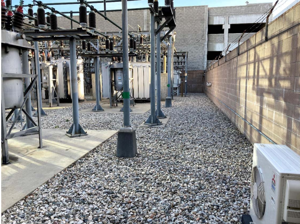
Photo 7: The yard area was mostly gravel with concrete equipment footings and walkways. The view is to the east from the southwestern corner.
