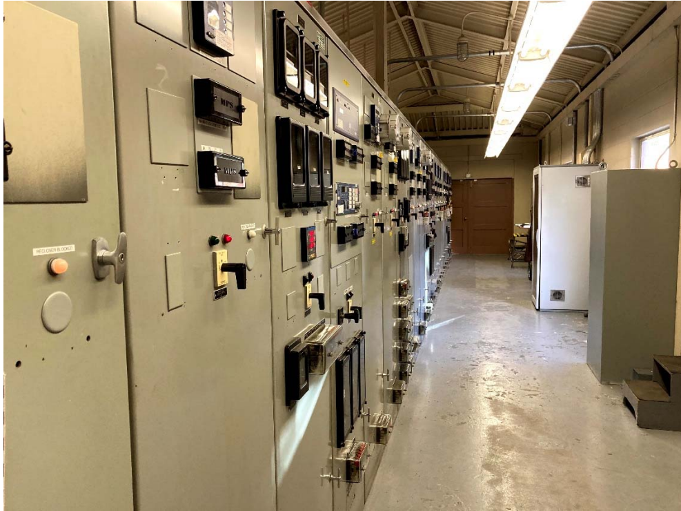
Photo 5: The view is from the southeastern corner of the control room to the north.
