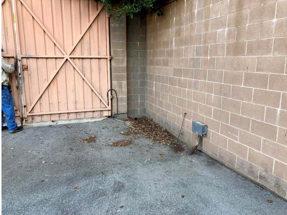
Photo 11: A stormwater drain was blocked with leaves in the northeastern corner, inside the vehicle access gate.
