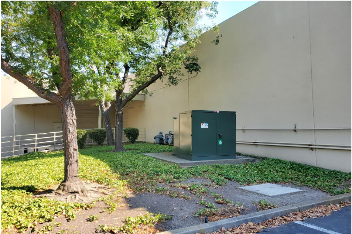
Photograph No. 17: One of two pad-mounted electrical transformers located on-site.
