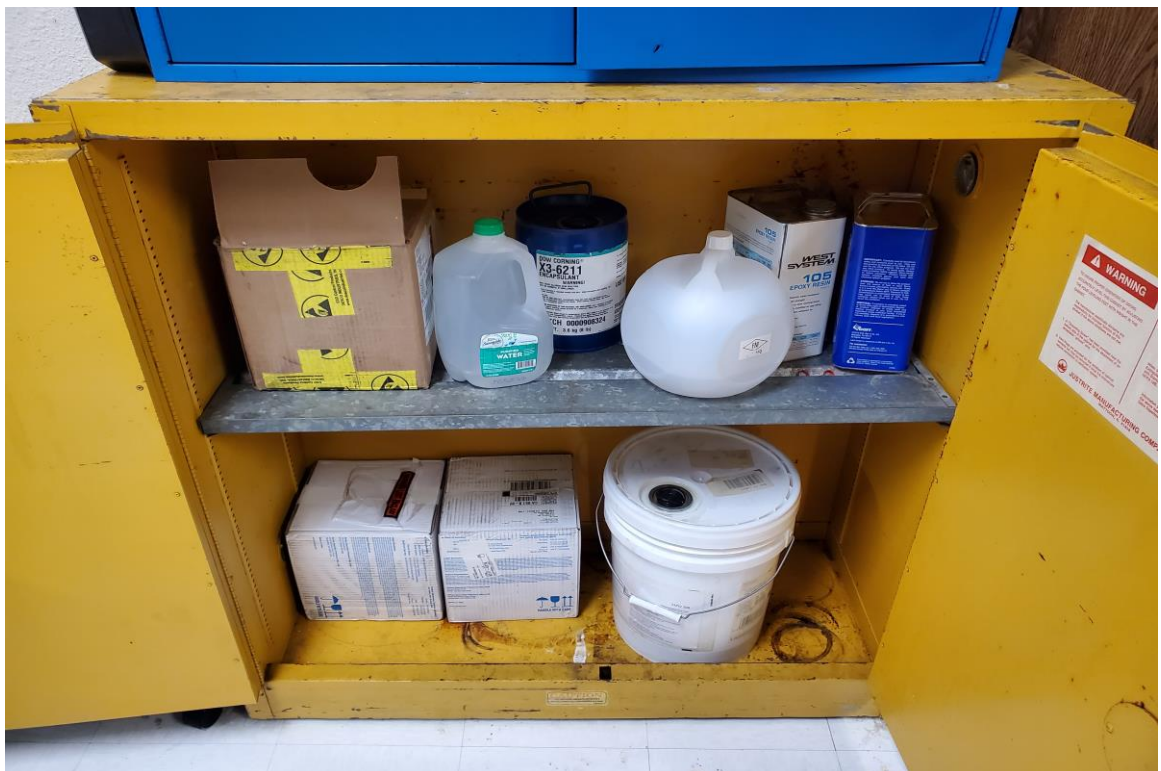
Photograph No. 8: One of three fire cabinets with small quantities of chemicals used by Silitronics.
