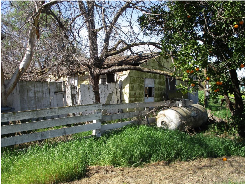
Figure 35. Photograph showing the south and east elevation of the ca. 1920 cottage, facing northwest.
