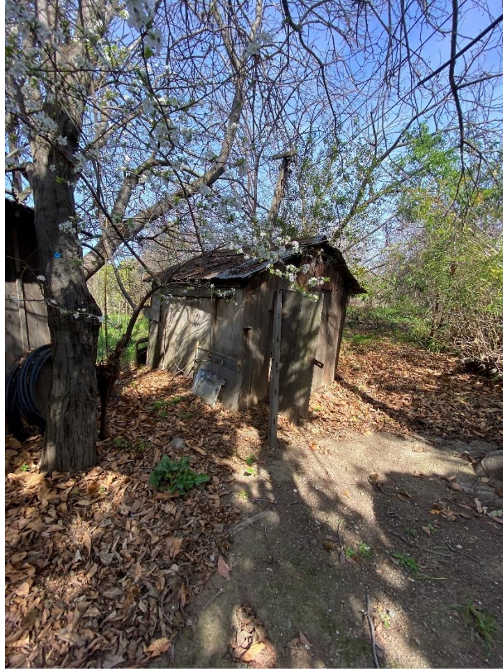
Figure 54. Photograph showing the south and west elevations of the ca. 1930 pump house.
