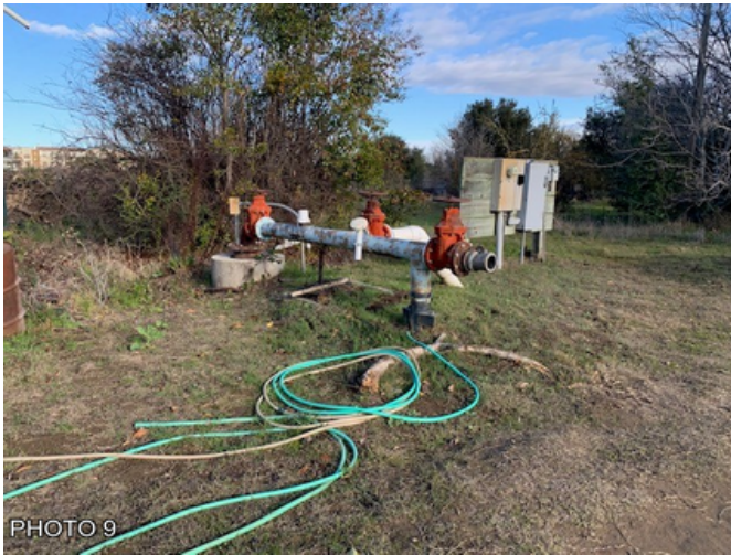
PHOTO 9 VIEW OF WATER SUPPLY WELL AND PUMP
