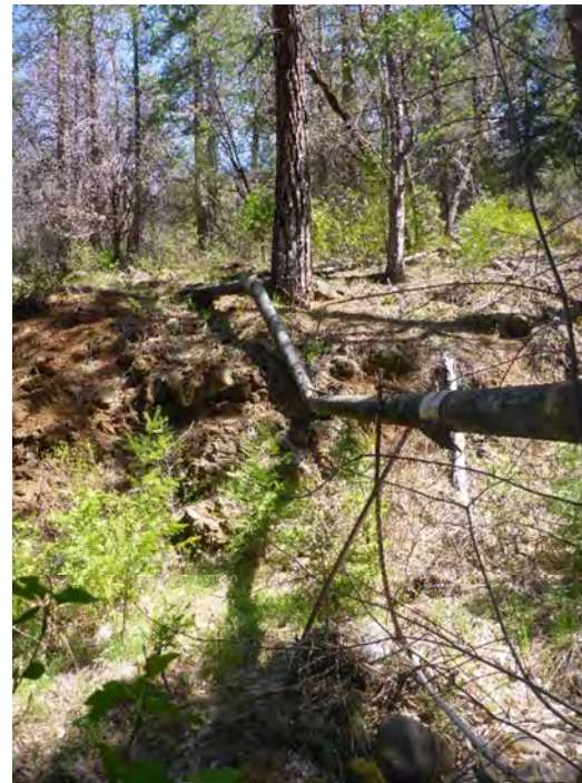
Photo 4.10.3. Transmission Main Facing the North Side of the Creek.
