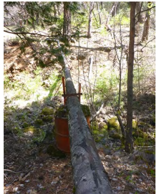
Photo 4.10.1. Transmission Main on South Side of Paynes Creek.
