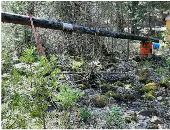
Photo 2. Transmission Main over Paynes Creek to the Well.
