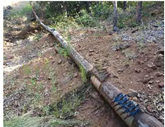
Photo 3. Transmission Main with Repair Clamps
