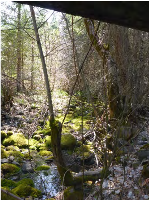
Photo 4.10.2. Paynes Creek Channel Under the Transmission Main.
