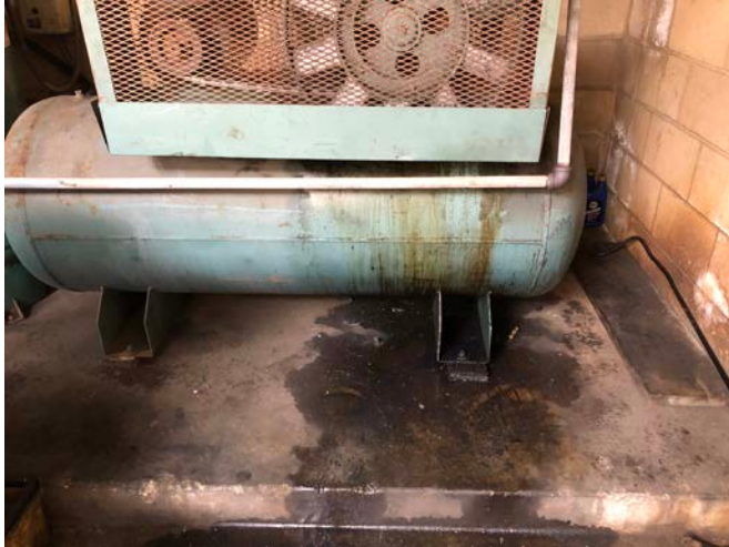
19. Floor staining near air compressor equipment
