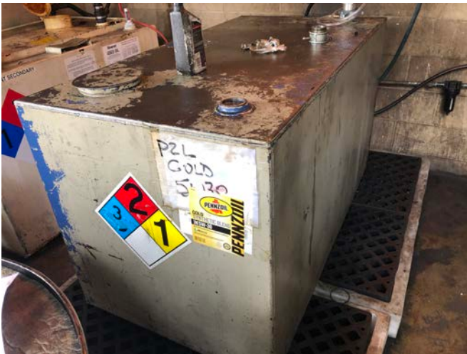
15. 240-gallon aboveground oil tank
