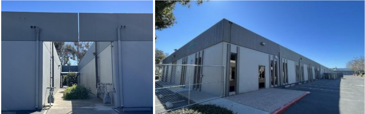
Figure 51. Corridor between buildings B and C (left) and Building C, east corner (right).
