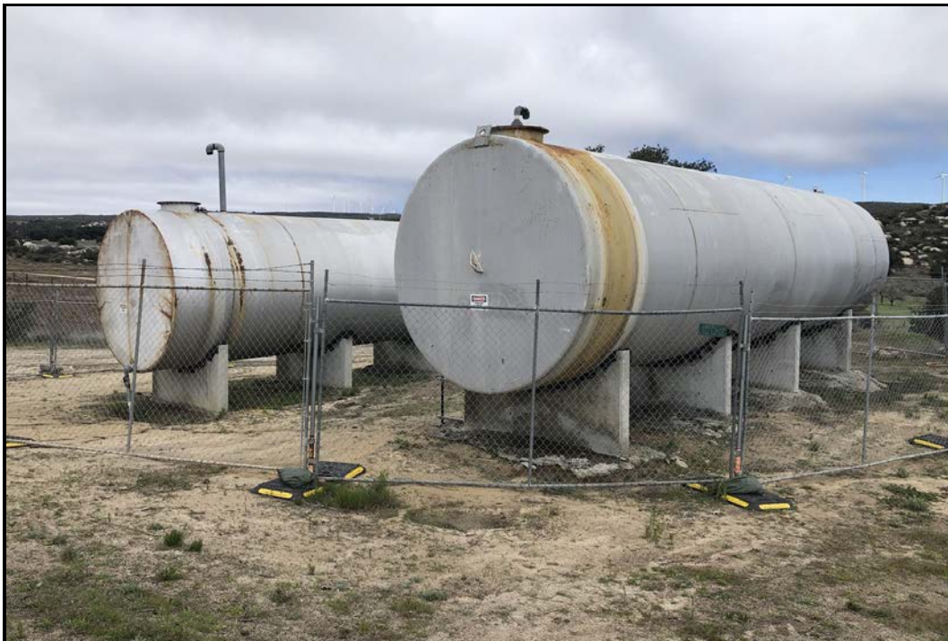
PHOTOGRAPH 2 Current Water Storage Tanks, Looking North
