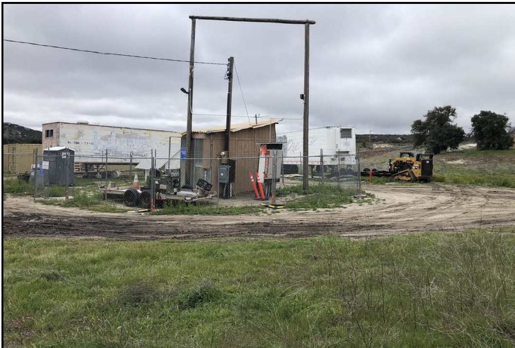
PHOTOGRAPH 4 Main Live Oak Springs Water System Utility Area, Looking South
