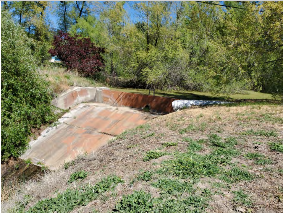
Photograph 10: Northwest-facing view of the concrete dam and spillway at the southern end of freshwater Pond 1 in the southern portion of the project site. The concrete dam has formed Pond 1 within Campo Creek and has contributed to the formation of the freshwater marsh within the southern extent of Campo Creek (due to the ponding of water).
