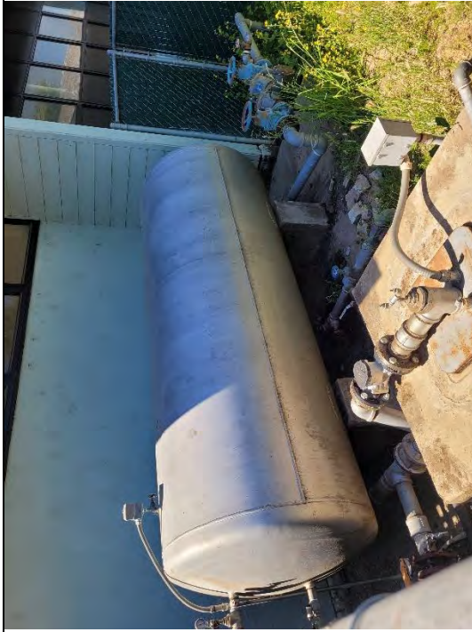
Photo No.7 – Reported 3,000-gallon Water Tank, located approx. 150-foot north of the Project Site.
