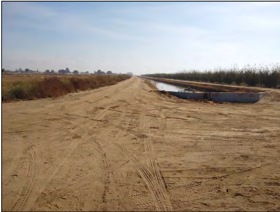
Figure 4. Overview of proposed pipe corridor along dirt road right-of-way between Road 164 and Woodville Road, looking east.
