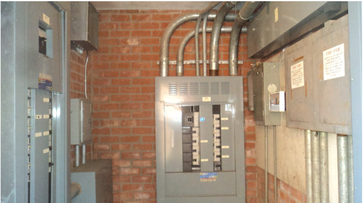
Photograph 14 – Utility room located in central portion of subject property.
