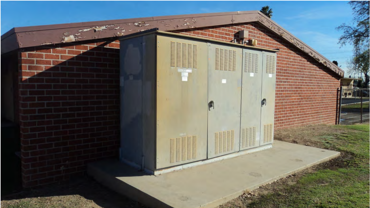
Photograph 11 – Looking north toward pad-mounted transformers on the eastern portion of the subject property.
