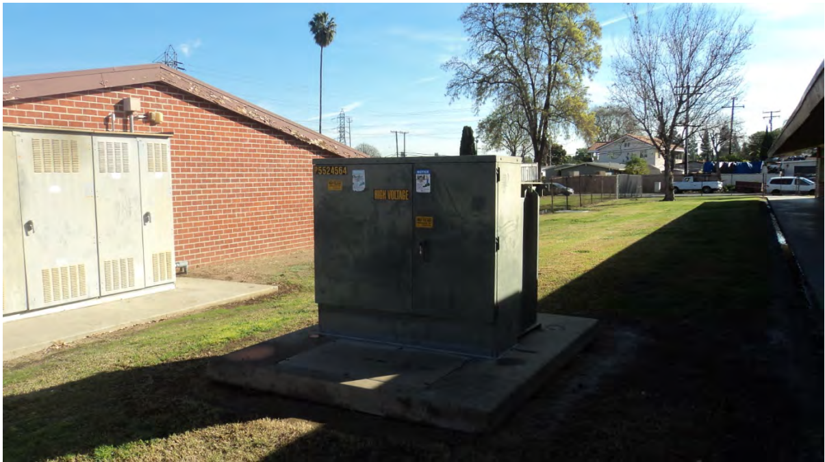
Photograph 20 – Pad-mounted transformer in northern portion of subject property.
