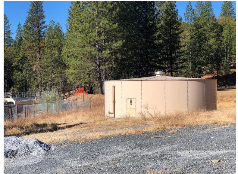
View of existing sewer storage tank in foreground and sewer treatment tank in the background. Both to be retained.
