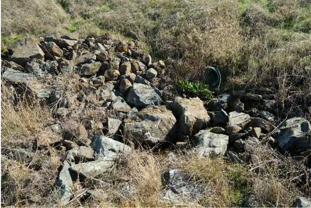
Photo 11. Closeup of culvert and rockpile north of the stormwater basin, facing southeast.
