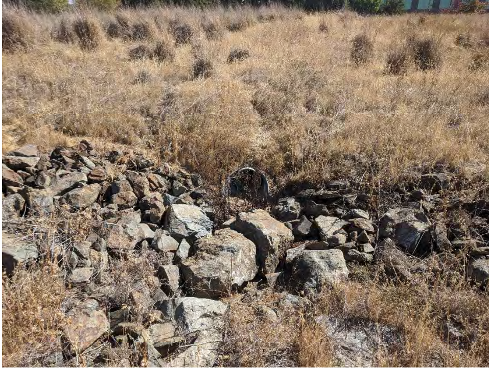
Photo 5: View of the culvert outfall that drains stormwater runoff into the constructed depression. Photo taken October 13, 2021.
