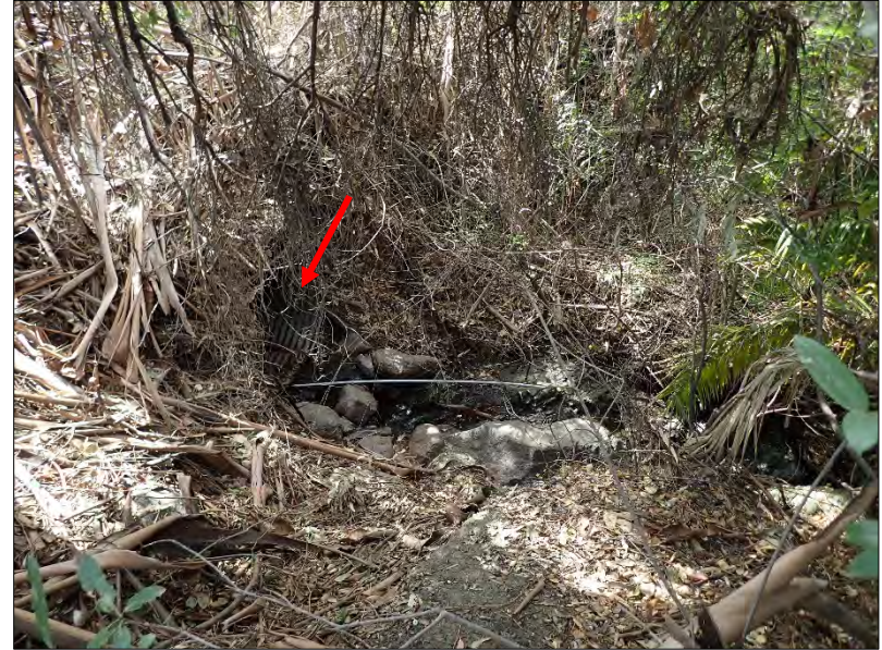
Photo 6: View southeast at culvert outfall (arrow) below the Iris Street cul de sac to the drainage flowline at the bottom of the eucalyptus dominated ravine. 4/17/2021
