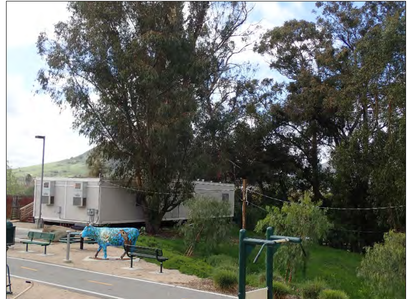
Photo 2: View southwest at eucalyptus removal "north" area around construction trailer at the edge of the parking lot and top of slope above railroad tracks. 4/17/2021
