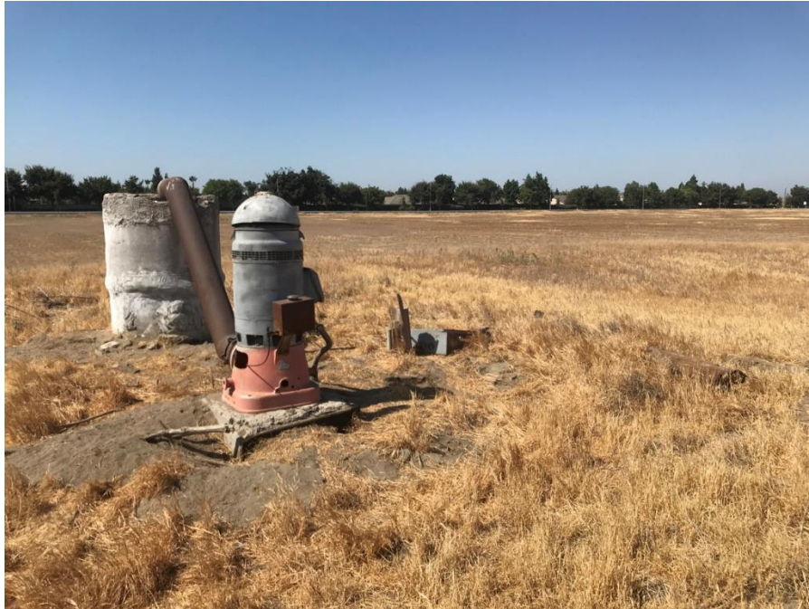
Photograph 11: Pump and well in the southeast area of Project site. GPS Coordinates: 36.241674, 119.323374, facing south southwest. Photograph taken by Shannon Gleason on July 8, 2021.
