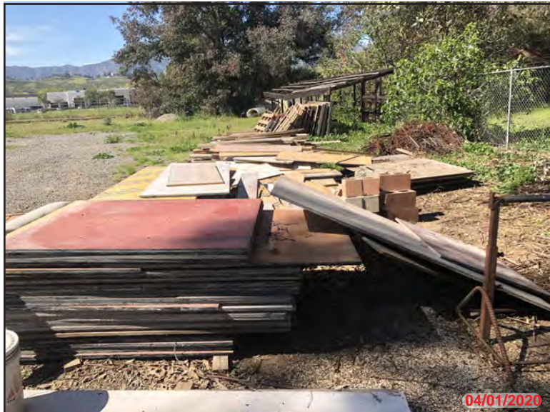
Photo 27- Exterior APN: 289-220-005, miscellaneous construction debris stacked and scattered south of the storage/maintenance shed.
