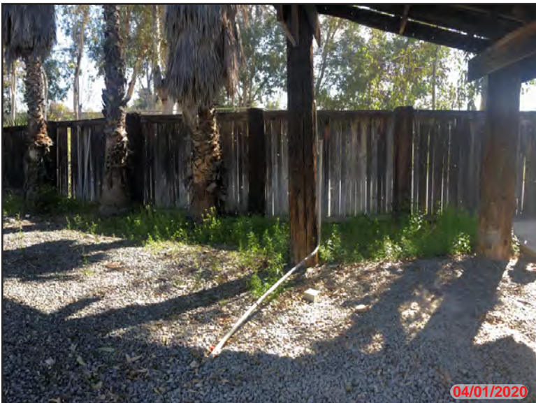
Photo 7 - Exterior APN: 289-220-003, a wood fence running N/S along the eastern Target Property line near the northeast corner of wood canopy (in frame.)
