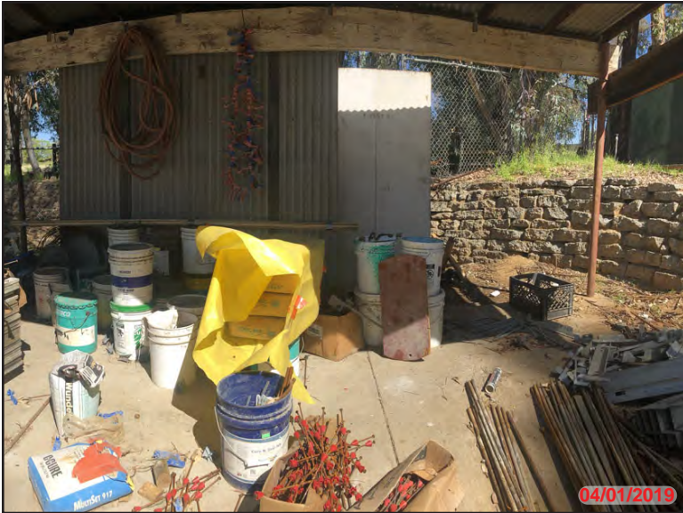
Photo 21 - Exterior APN: 289-220-004, Construction related debris and supplies of a nonhazardous material nature. This material consist of biodegradable sealant iron rods, a bag of cement and miscellaneous related material.
