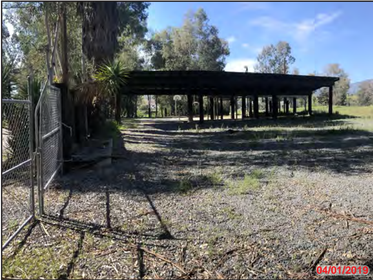
Photo 5 - Exterior APN: 289-220-003, looking S.W. toward Collier Ave. from N.E. corner of parcel with wood framed canopy in view at top of frame. The canopy is situated directly east of the previous residential structure.
