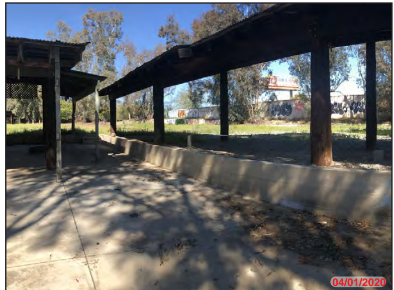
Photo 8 - Exterior APN: 289-220-003, from northwest corner of wooden canopy looking northwest with retaining wall in approximate center frame across demolished former residential structure pad area.
