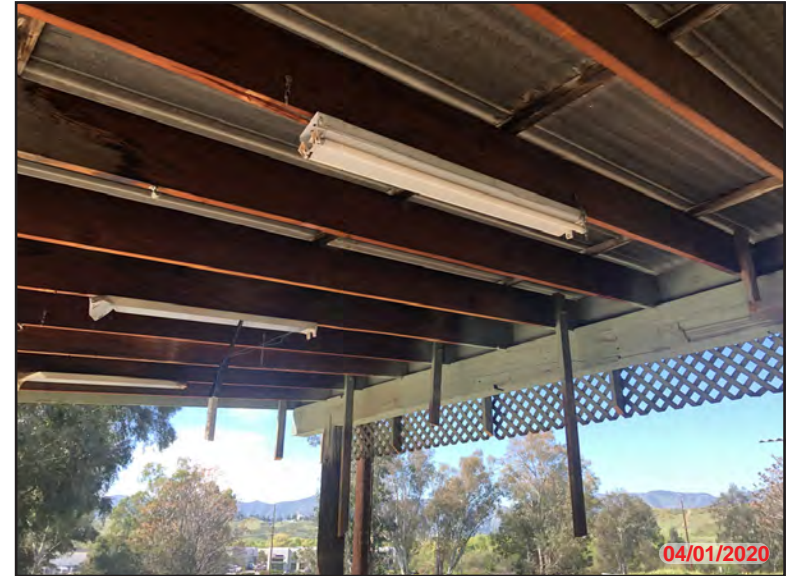
Photo 10 - Exterior APN: 289-220-003, under canopy with top interior ceiling and damaged florescent lighting fixtures in view. Broken light fragments are captured in photo # 12.
