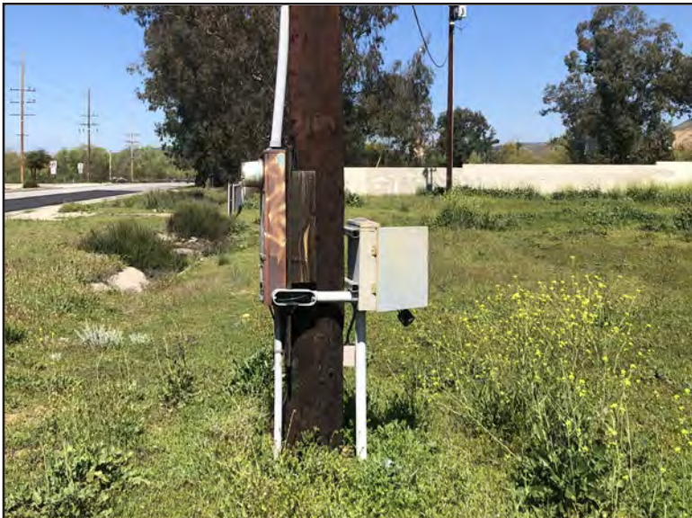
Photo 47 - Exterior APN: 289-220-006, electrical power supply control box. Appears to be to supply electricity to the well pump in photo 46.
