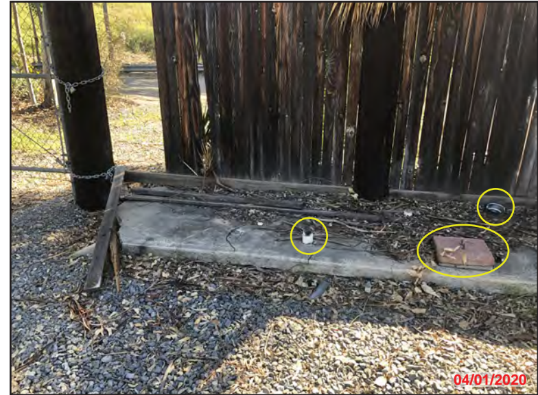
Photo 6 - Exterior APN: 289-220-003, near N.E. parcel P.L. with concrete electrical utility slab in view. PVC conduit extending from top of slab and a brick access cover are visible .
