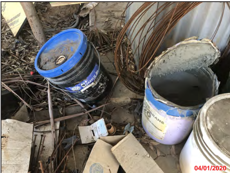
Photo 23- Exterior APN: 289-220-004, 5-gallon container of hydraulic fluid. The material while sealed in the container does not represent an REC, it should be disposed of properly off-site during demolition operations.
