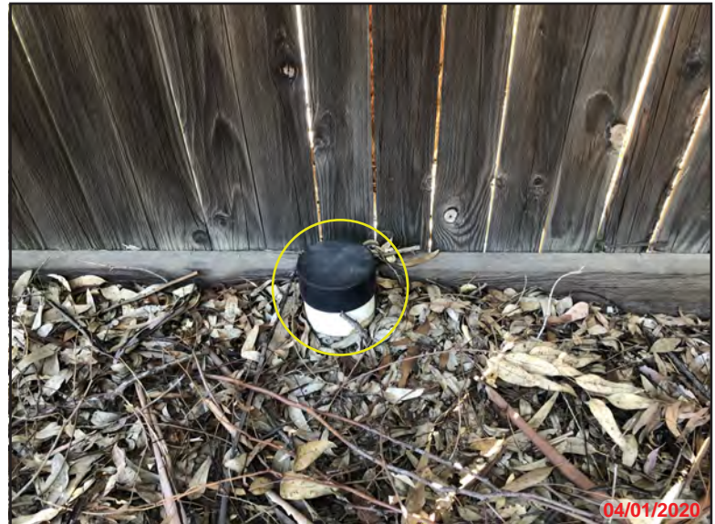
Photo 16 - Exterior APN: 289-220-003, Easterly Target Property adjacent to El Toro Road. PVC conduit, unknown purpose.
