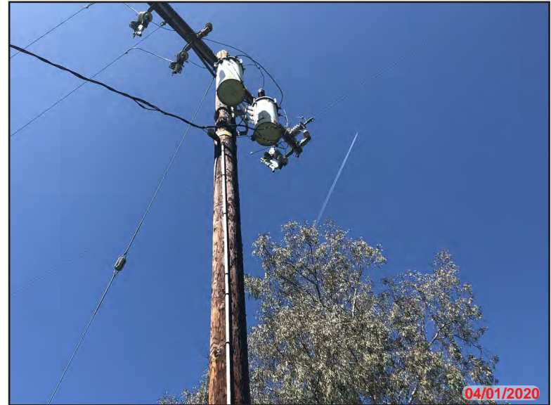
Photo 48 - Exterior APN: 289-220-006, Telephone pole with transformers located at the northwest area of the Target Property.
