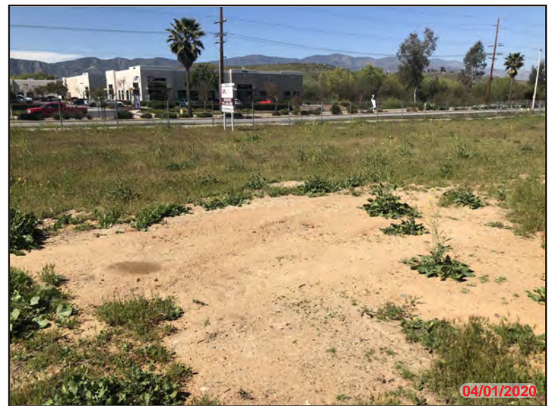
Photo 44 - Exterior APN: 289-220-006, apparent excavation pit. No records are available to indicate that the excavation pit is related to an underground structure removal.
