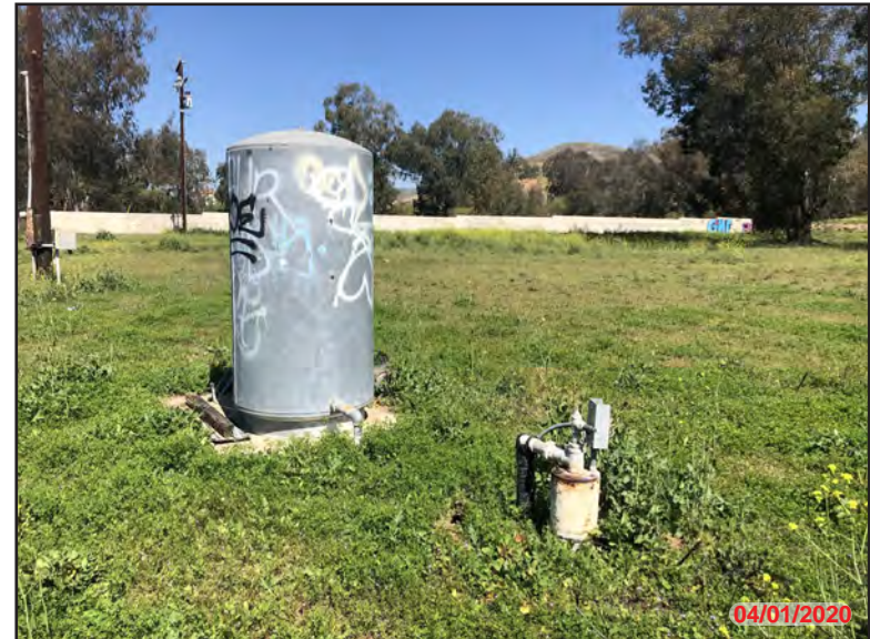
Photo 46 - Exterior APN: 289-220-006, abandoned water well tank and well head with associated electrical and plumbing apparatus.
