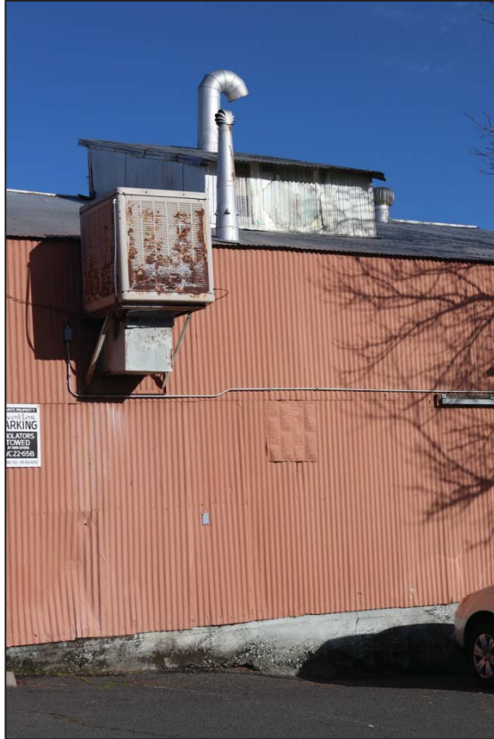
Photo 41: South elevation, mechanical equipment detail
