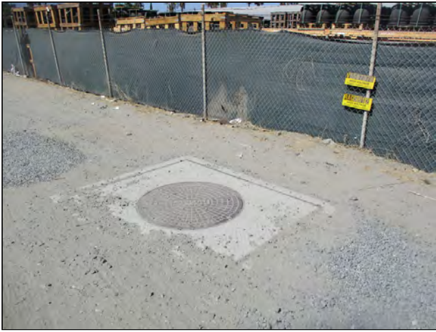
Edison utility vault on Project Area.
