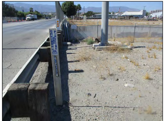
Gas pipeline marker at Temescal Wash and All American Way
