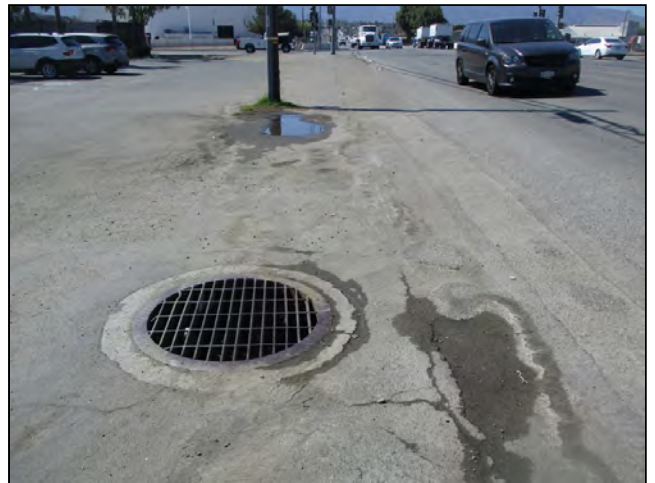
Storm water drain at Corona Auto Parts
