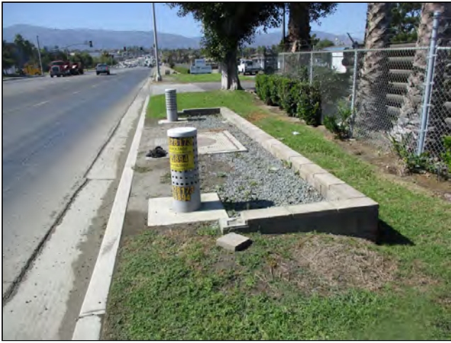
High voltage electrical on north side of Project Area.
