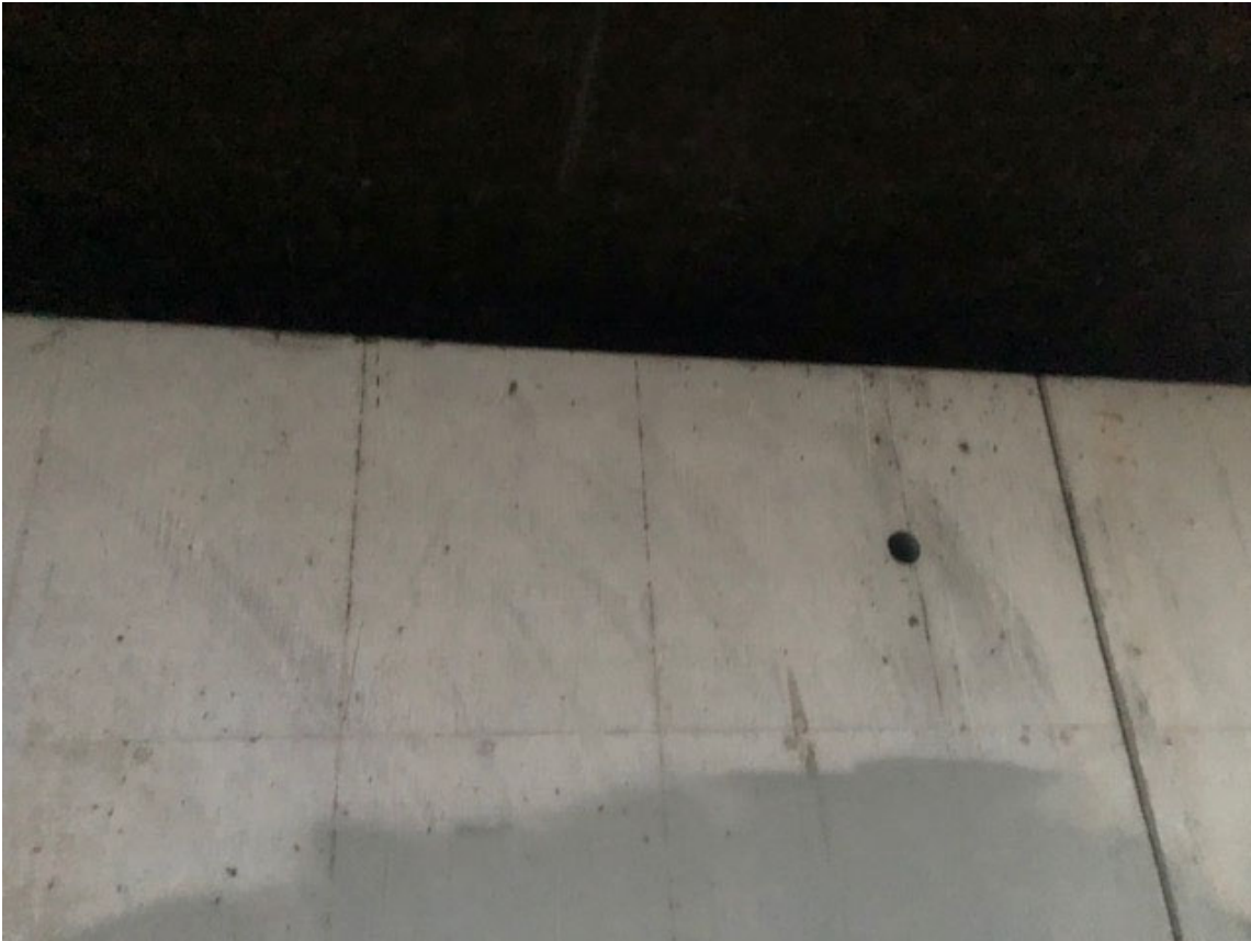
Photo 6. Showing sealed joint in the wash, which would prevent bats from roosting.
