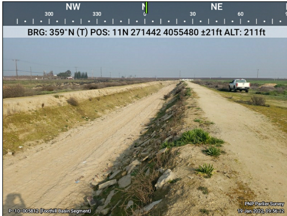
Figure 2. P-10-005812 at location of Foothill Basin pipeline tie-in.
