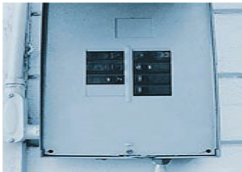
Electric Breaker Panel
