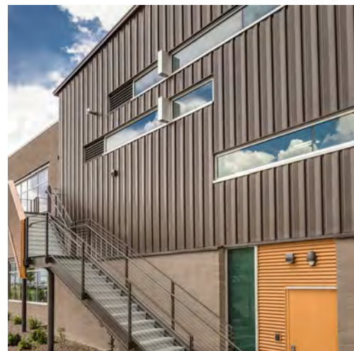
A "WING" ADDITION EXTERIOR CLADDING, TYP: MBCI "AVP" FLUTED METAL PANEL IN "SLATE GRAY" FLUTED METAL PANEL
