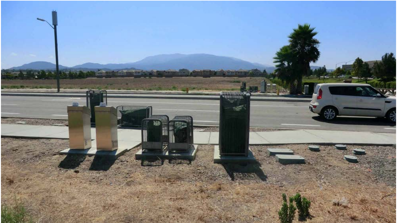
Facing southeast across Wolf Valley Road, bisecting the subject site, shown in foreground and background; typical utility access cabinets for water, street signage, telecommunications.
