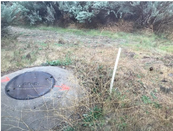
Sewer Manhole Indicating Direction of Flow (North); Under Western Boundary of Target Property
