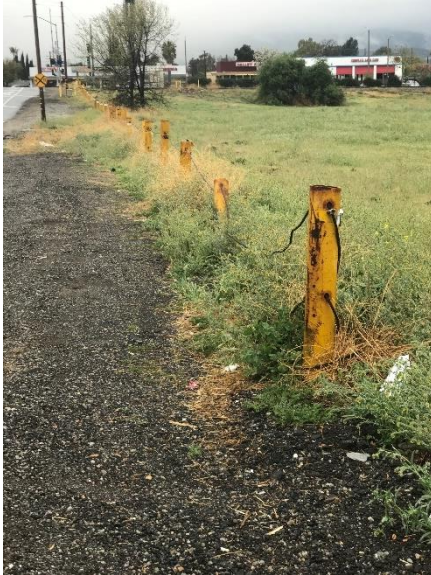
Facing West – Cable Fence Along 13 th Street Severed (Allowing Unobstructed Access to the Property)
