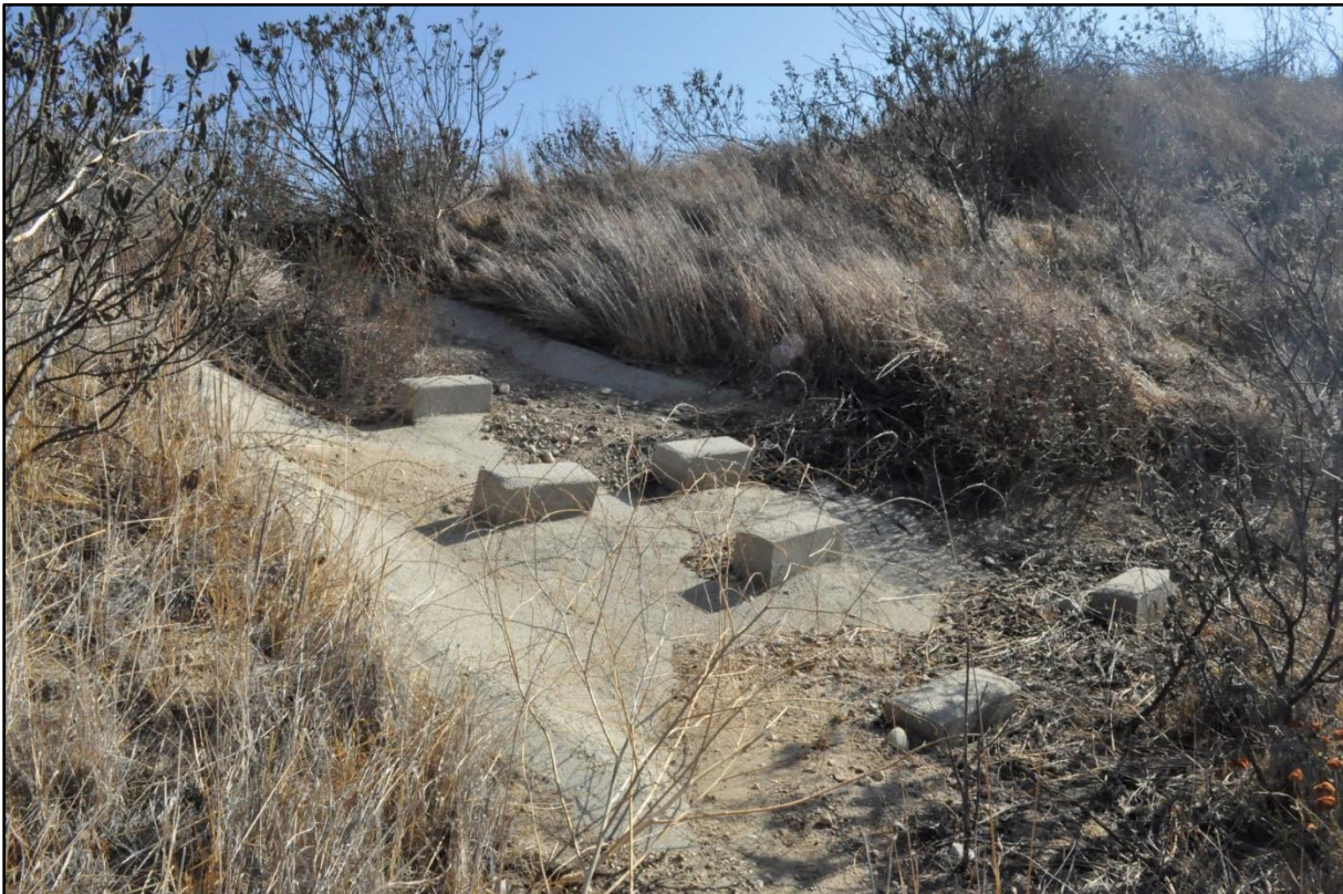
Figure 16. View towards the northeast of water aeration and remnant aqueduct structures on northern hillside.
