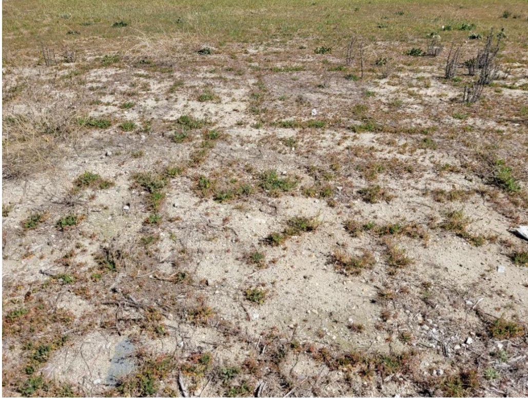
Figure 15. View towards the east of the brush and gravel. The obscure brush lines is due to the brush growing above the asphalt that was laid under the gravel
