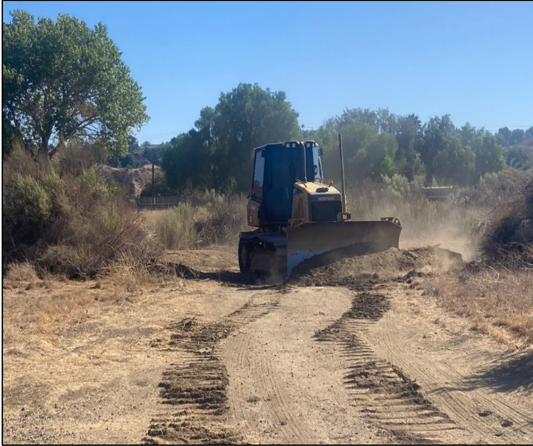
Figure 25. View of large scraper creating path for boring machines and removing vegetation
