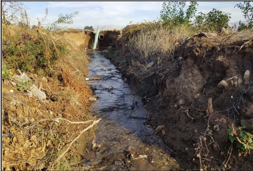
PHOTOGRAPH 4 View of Earthen Channel Section of Jurupa Ditch Below Concrete V-ditch Section Looking North
