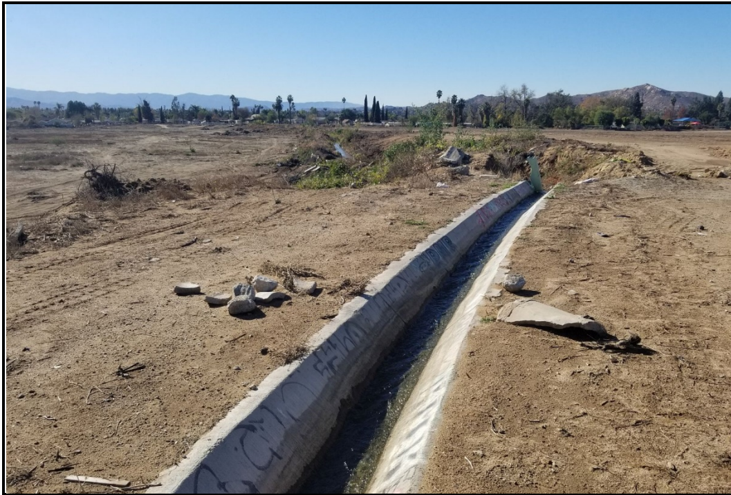
PHOTOGRAPH 3 View of Concrete V-ditch Section of Jurupa Ditch Above Transition to Earthen Channel Looking South
