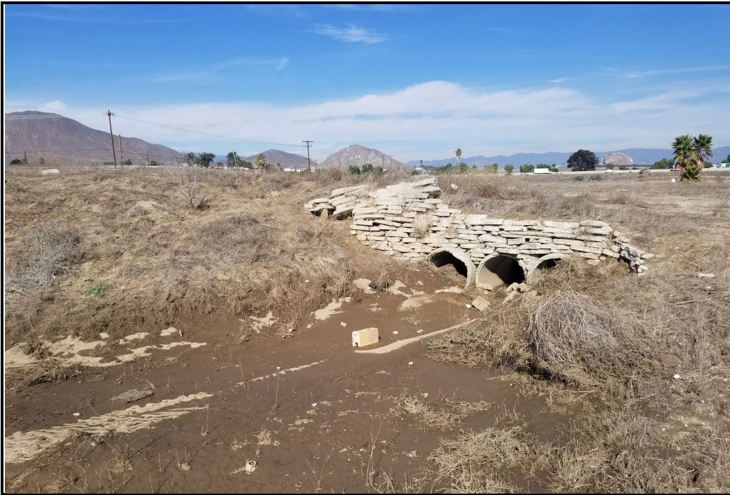
PHOTOGRAPH 9 View of the Un-named Drainage Below a Dirt Road Culvert Looking North
