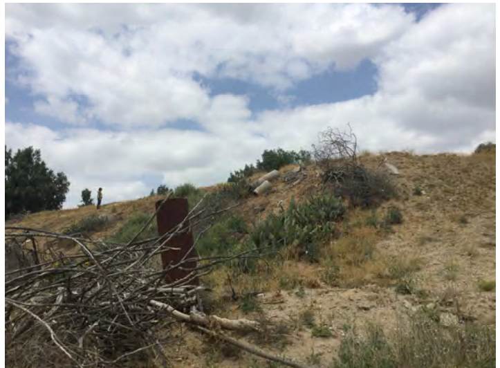
Figure 2. Overview of the northeastern section of CA-RIV-5513H, showing concrete piping sliding downslope of its original position. Photo facing north.
