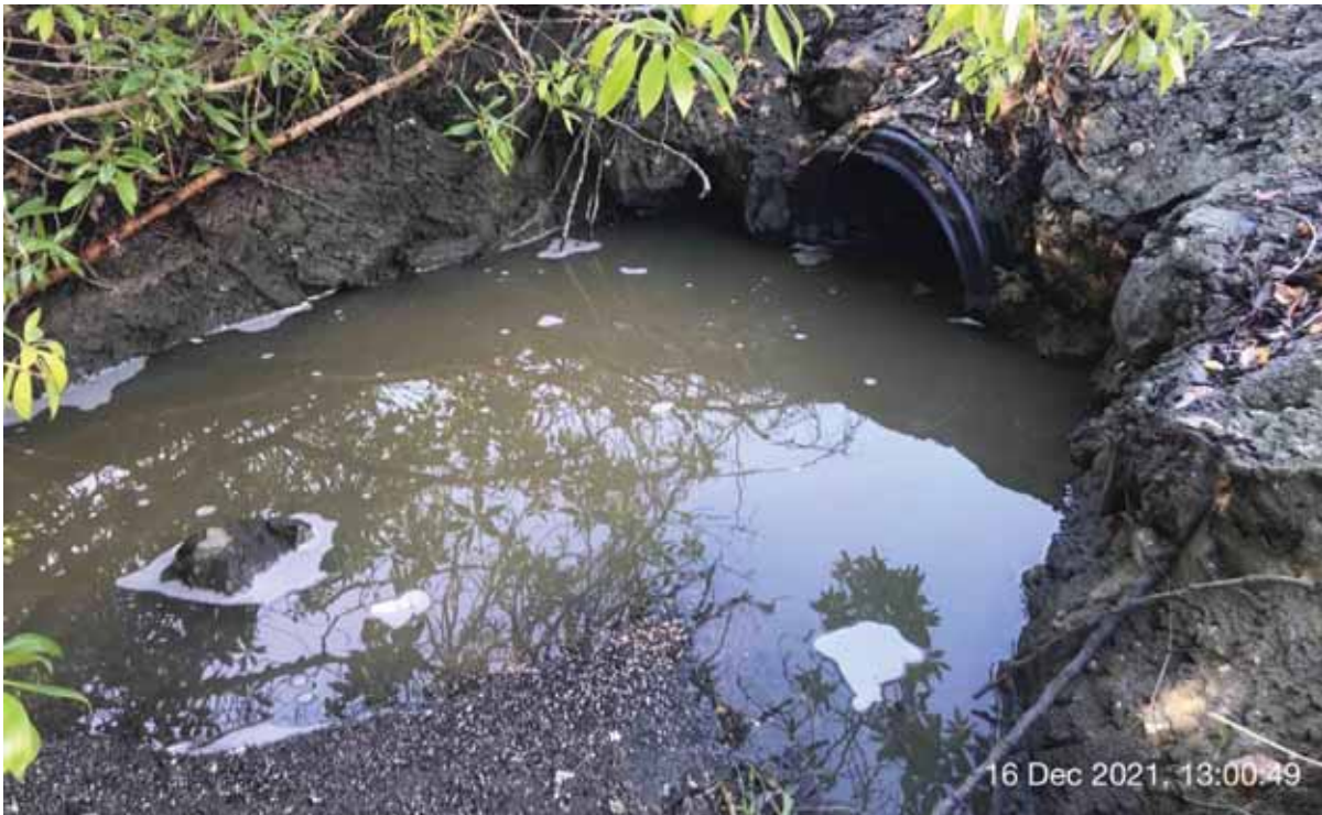
Photograph 10. View of the culvert that conveys water from beneath Pillar Point Harbor Boulevard to Pillar Point Harbor. The drainage is surrounded by several arroyo willows.
