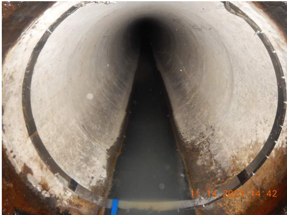
Monitored Southeast Inlet Pipe
