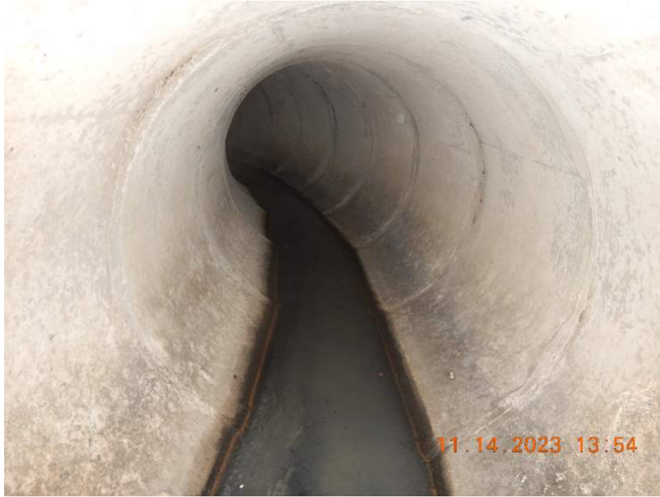
Northwest Effluent Pipe
