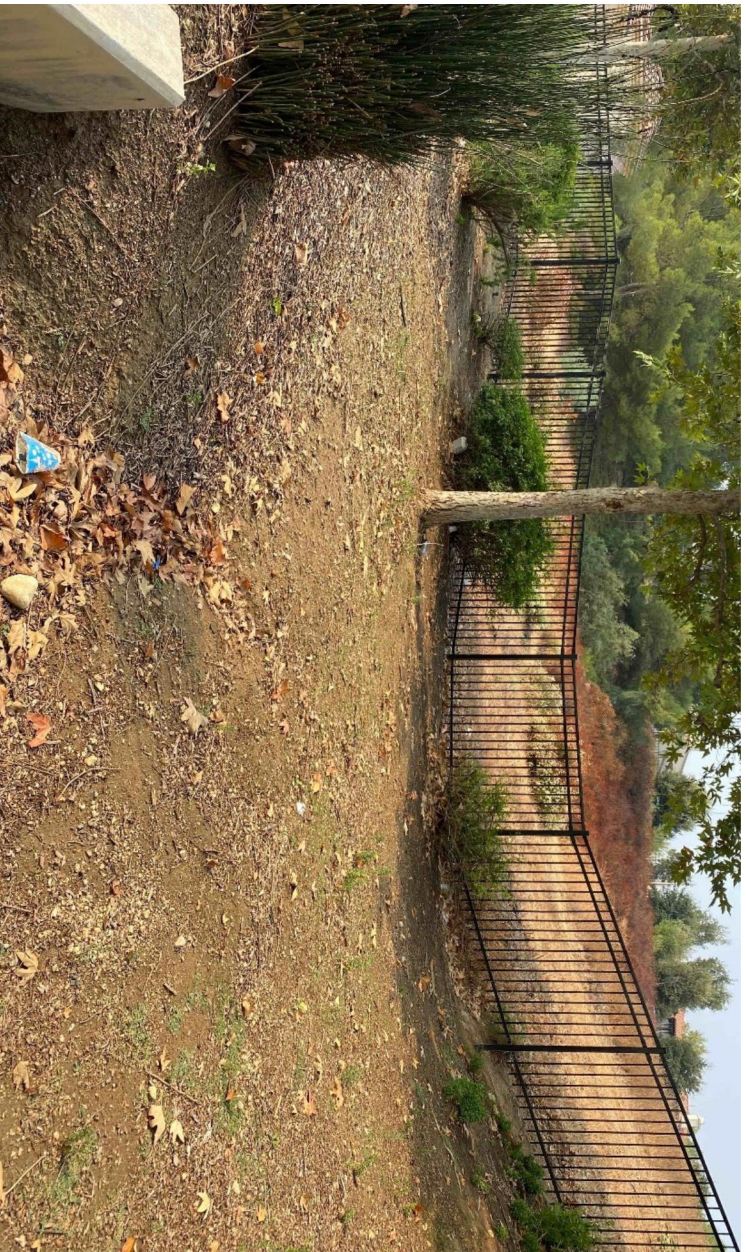
Photograph 8. Storm drain inlet northeast of proposed facility footprint within ornamental landscaping, view to the south. September 14, 2020.
