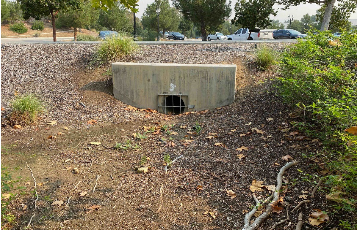
Photograph 3. View of existing storm drain, taken from eastern portion of project site facing northeast towards the McBean Regional Transit Center Park and Ride parking lot.
