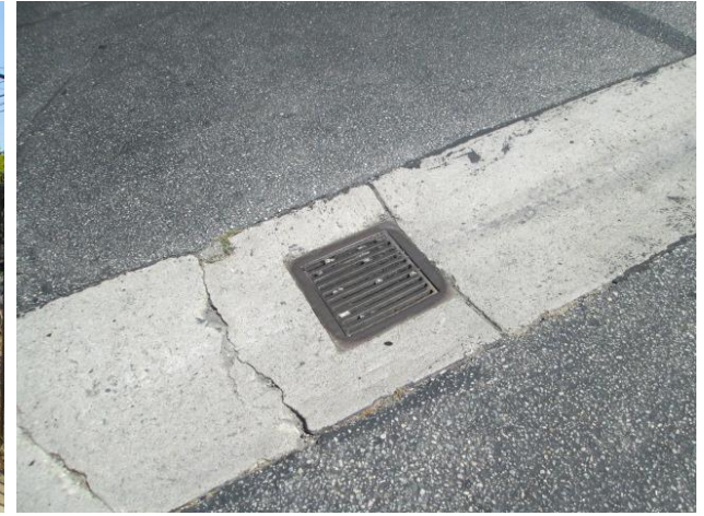
9. Typical area drain.
