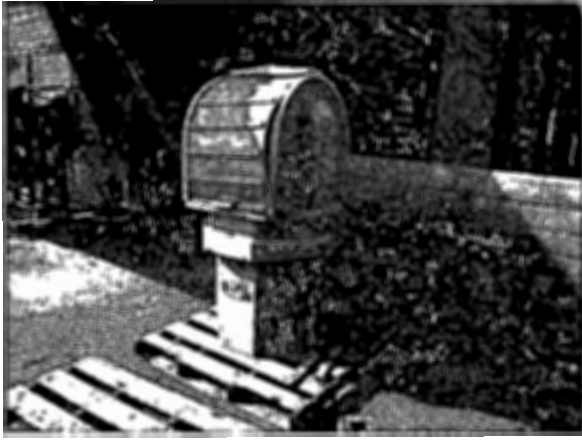
New oil containment
