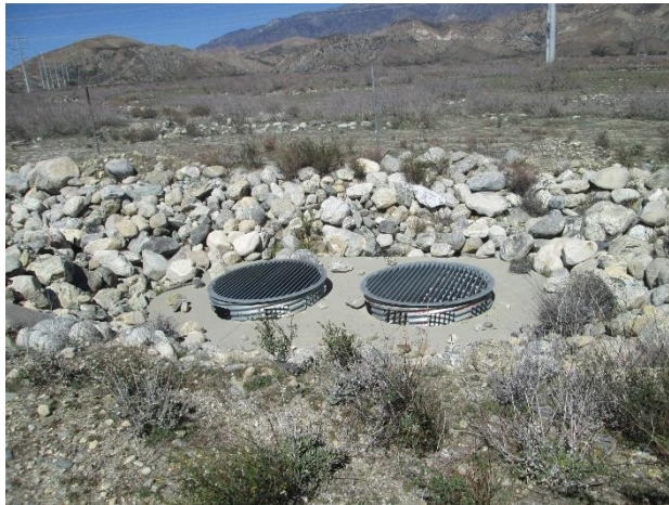
17. Typical drainage feature.
