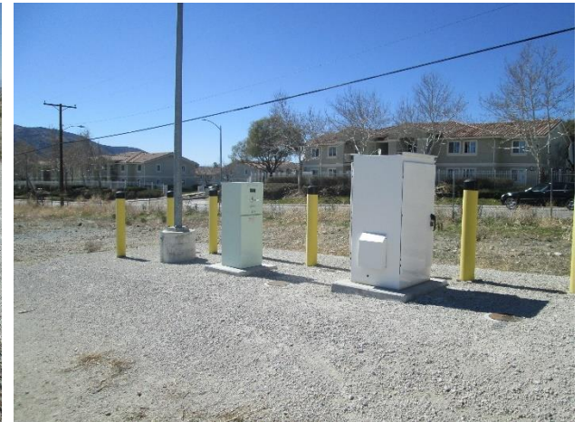
24. Utilities in the northwestern corner of the Site. Adjacent residences (west) are visible.
