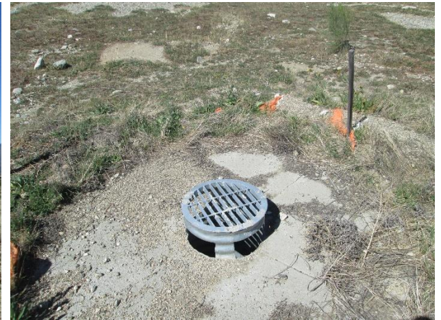
12. Typical drainage feature.
