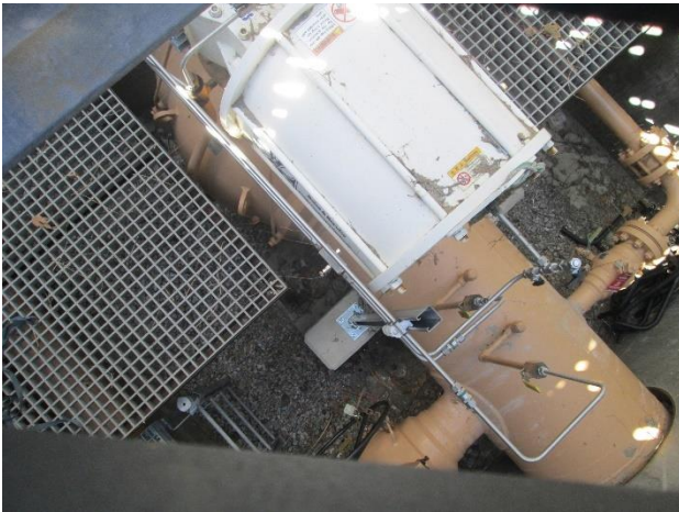
22. Gas pipeline vault and infrastructure.
