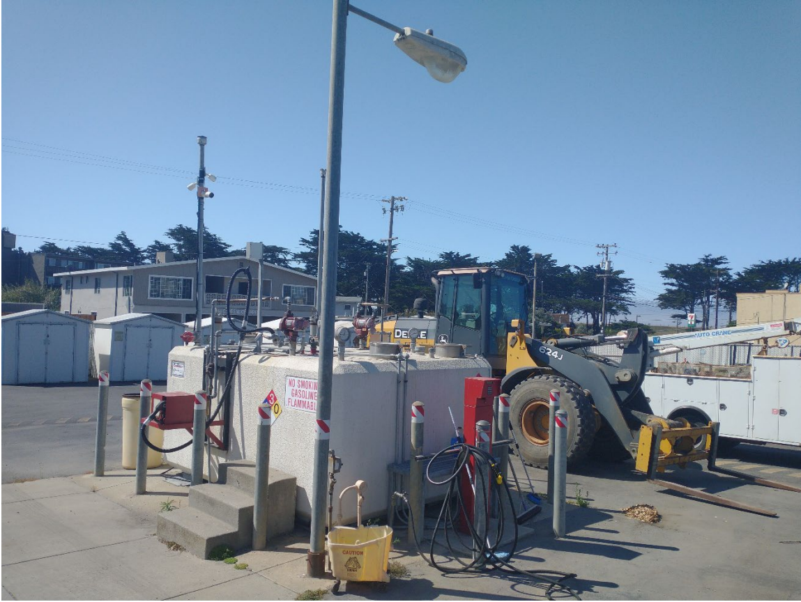
C-12. Fueling station in the middle of the laydown yard, at a distance of approximately 100-feet from the NCCWD Headquarters Complex’s buildings, view to the west-southwest. Photograph by Yarbrough Architectural Resources, Sept. 15, 2021.
