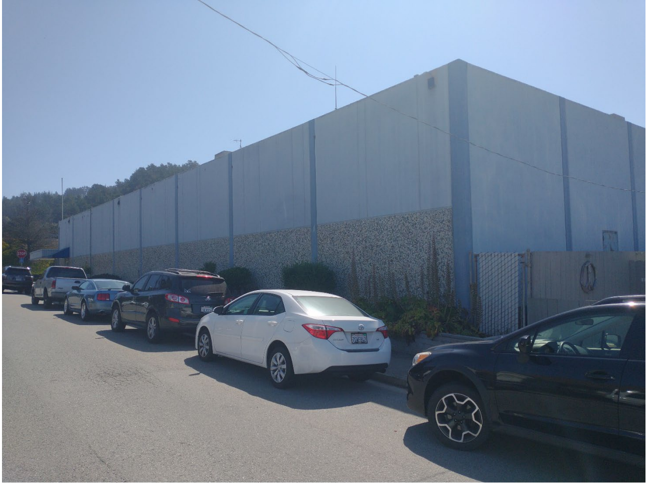
Figure 10 View of northwest corner of Building No. 2. Note the eight bays between nine posts on the north elevation built using tilt-up concrete construction. Photograph by Yarbrough Architectural Resources, Sept. 15, 2021.
