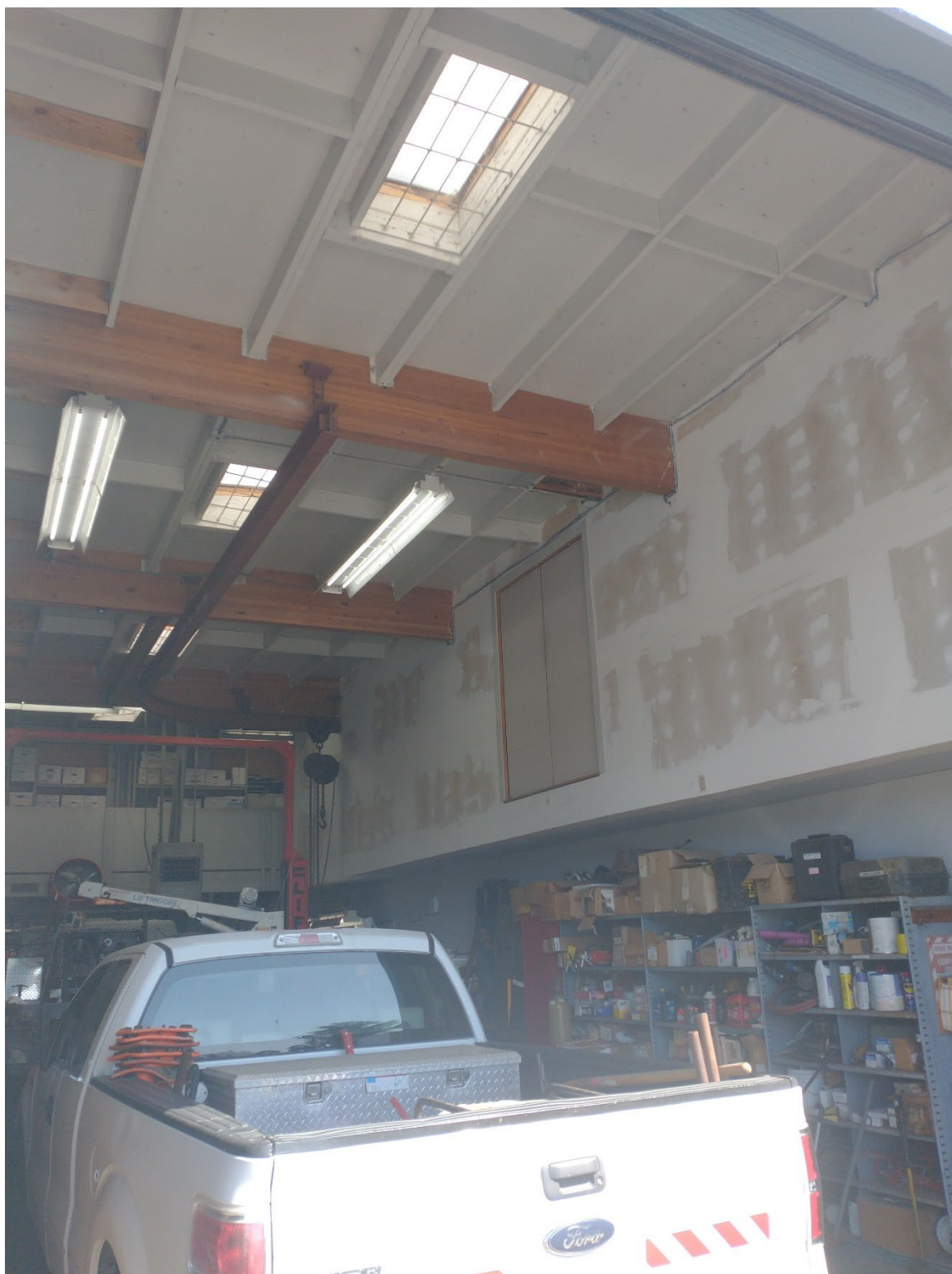
Figure 14 View north inside Maintenance No. 1. Note wood truss members, I-beam overhead-crane, and newer drywall, upper right, where office space was added to the eastern portion of the building. Photograph by Yarbrough Architectural Resources, Sept. 15, 2021.
