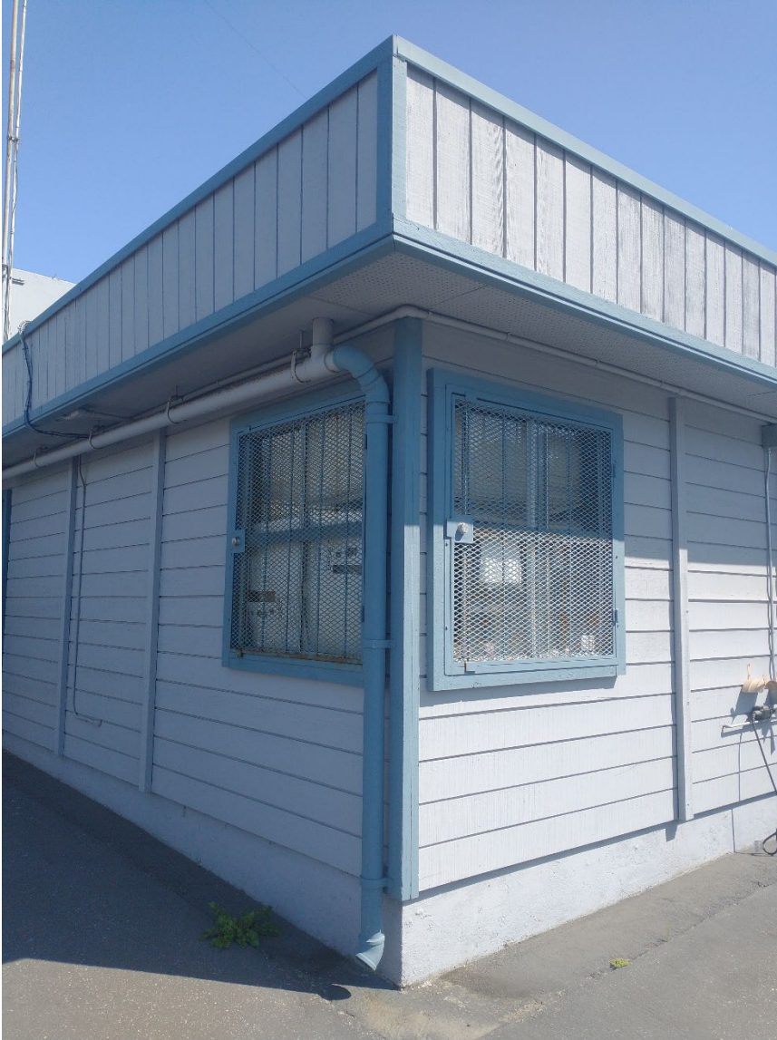
C-11. Southwest corner of the Administrative Building showing 1979 siding and windows with security expanded-metal screens, view to the northeast. Photograph by Yarbrough Architectural Resources, Sept. 15, 2021.
