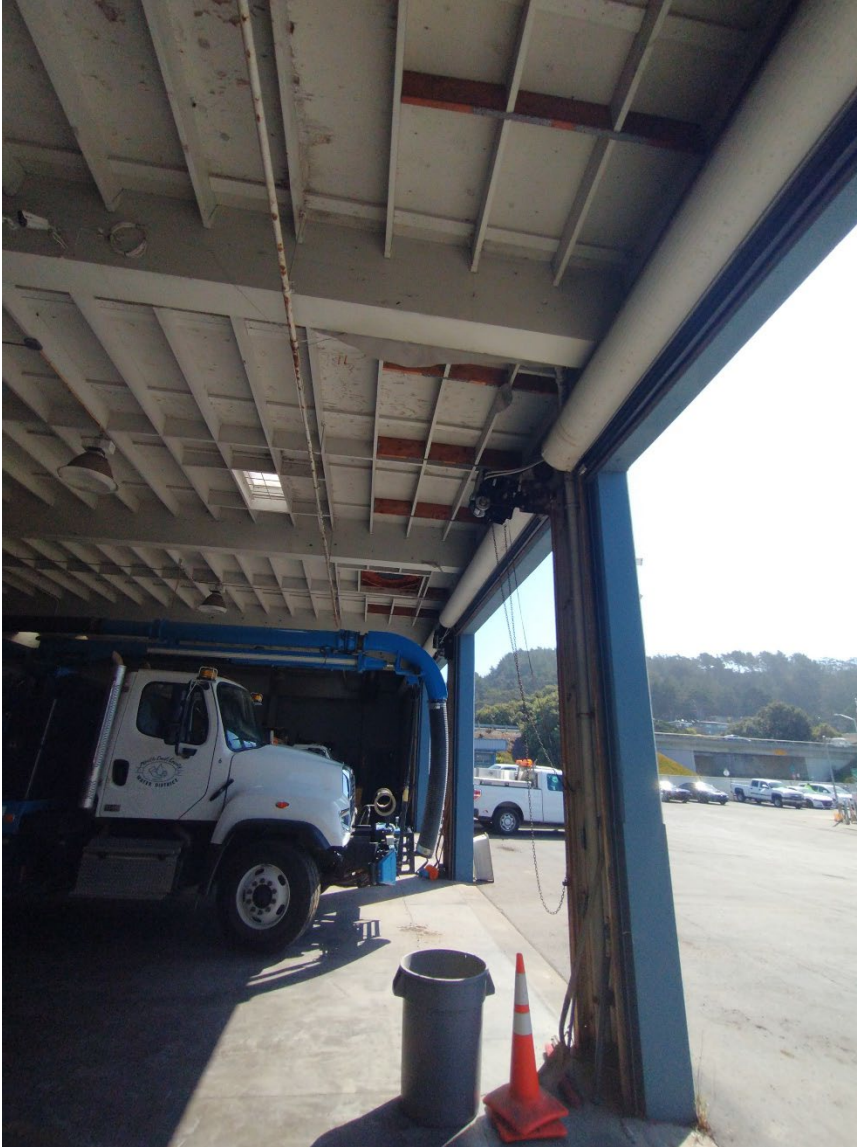
C-10. Inside garage bays of Building No. 2/Maintenance No. 2 looking east-southeast. Note retrofit rafter joist bracing (unpainted lumber) in the truss. Photograph by Yarbrough Architectural Resources, Sept. 15, 2021.
