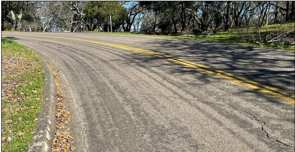
Bennett Ridge Road (Road ID: 66081B) - End of County Maintained Road to End of County Maintained Road, Santa Rosa. Length: 0.69 Mile. Treatment: Asphalt Overlay
