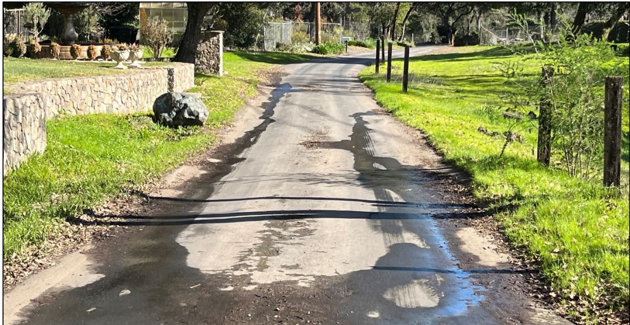
Bristol Road (Road ID: 66063) - End of County Maintained Road to Keiser Road, Kenwood. Length: 0.42 Mile. Treatment: Asphalt Overlay
