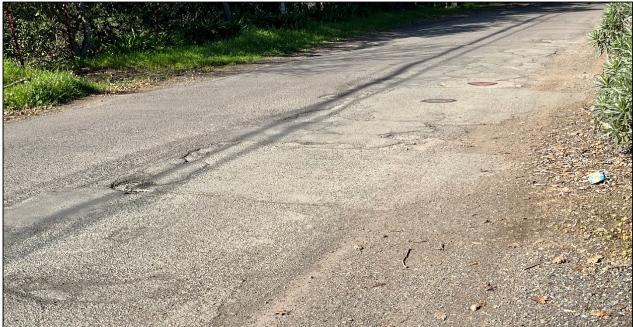
Castle Road (Road ID: 55044) - Seventh Street E to End of County Maintained Road, Sonoma. Length: 0.54 Mile. Treatment: Asphalt Overlay
