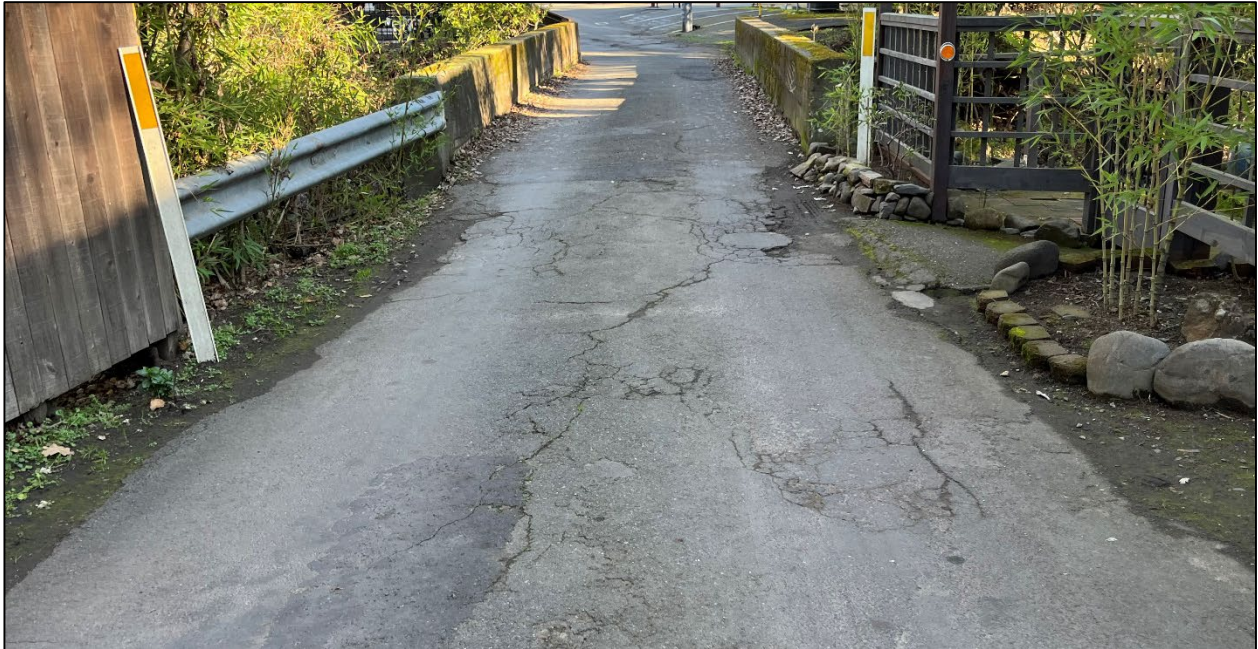
O'Donnell Lane (Road ID: 66048) - End of County Maintained Road to Arnold Drive, Glen Ellen. Length: 0.33 Mile. Treatment: Removal and Replacement of Asphalt Concrete; Asphalt Overlay.
