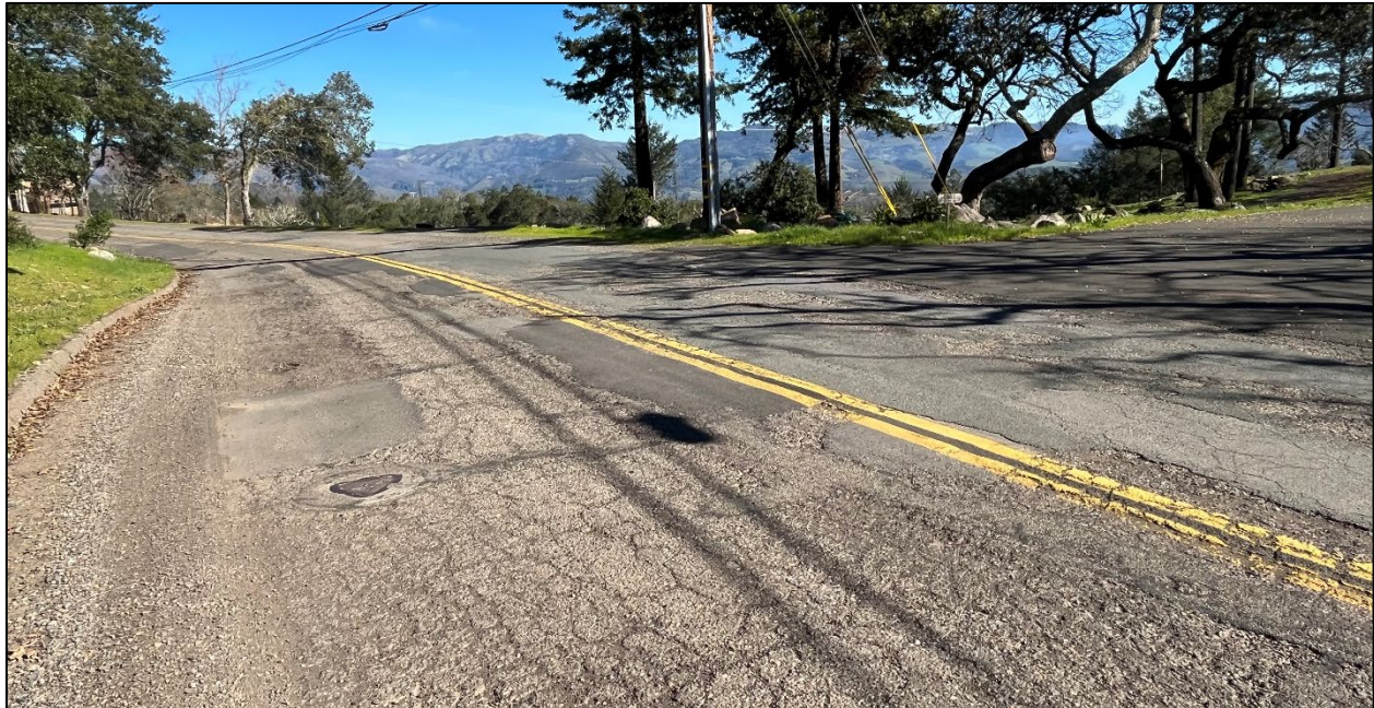
Bardy Road (Road ID: 66082) - Old Bennett Ridge Road to Bennett Ridge Road, Santa Rosa. Length: 1.35 Miles. Treatment: Asphalt Overlay
