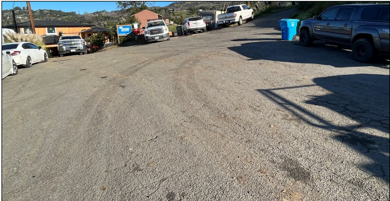
Donner Road (Road ID: 88060) - Wilshire Drive to Cul De Sac, Santa Rosa. Length: 0.29 Mile. Treatment: Asphalt Overlay
