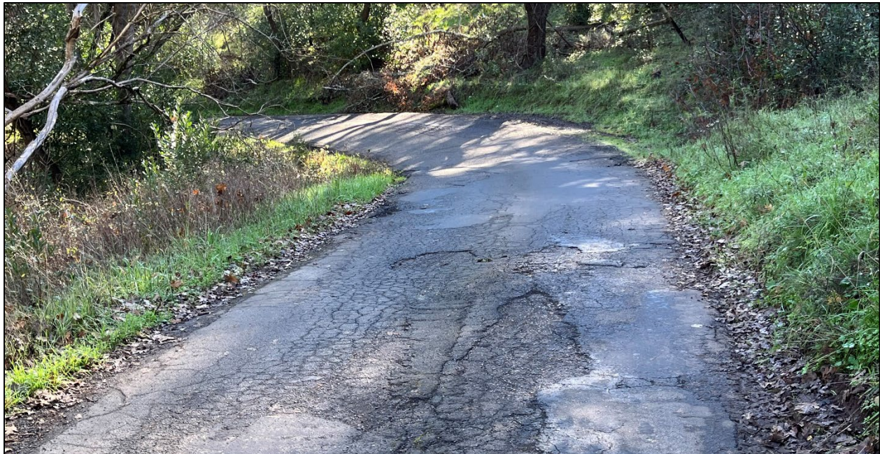
Kennilworth Avenue (Road ID: 76018) - End of County Maintained Road to Mervin Avenue, Kenwood. Length: 0.69 Mile. Treatment: Asphalt Overlay
