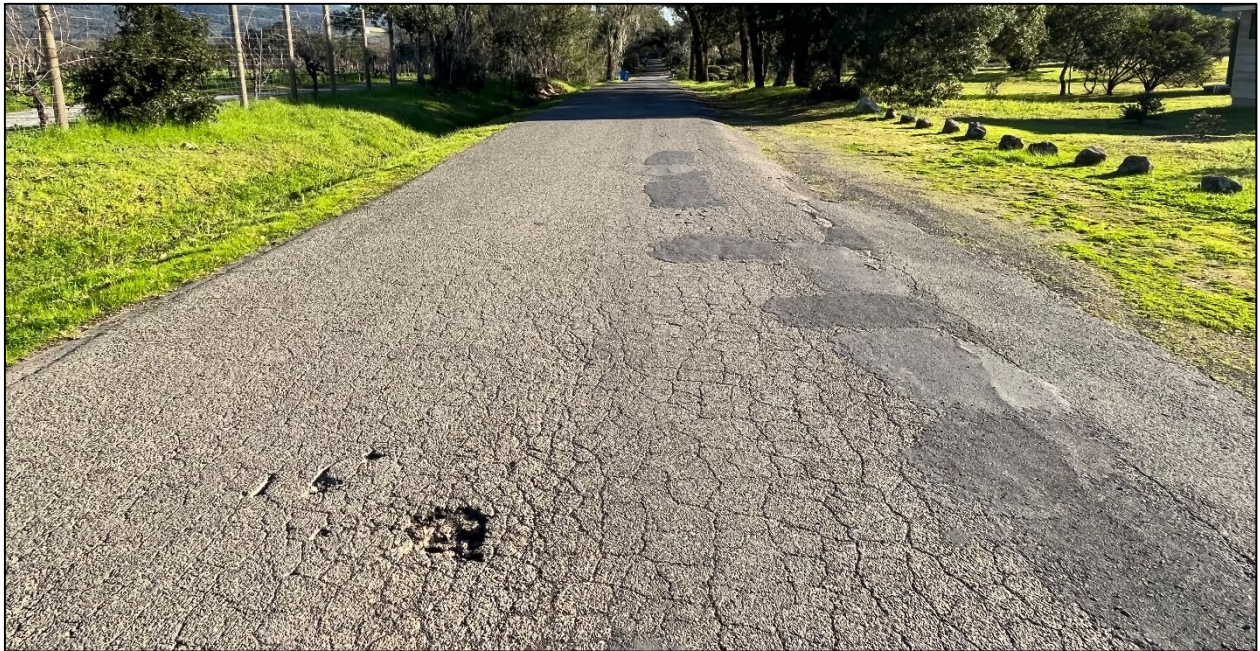
Henno Road (Road ID: 66049) – O'Donnell Lane to Dunbar Road, Glen Ellen. Length: 1.87 Miles. Treatment: Asphalt Overlay
