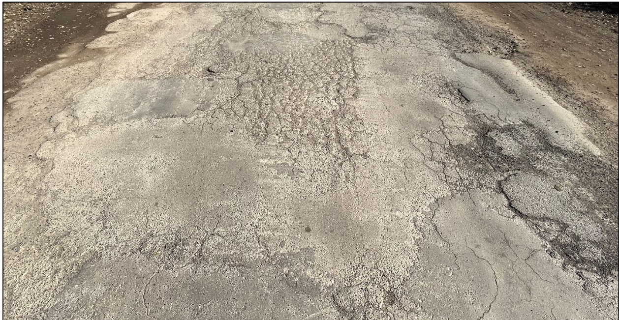
Thornsberry Road (Road ID: 55043) - End of County Maintained to Lovall Valley Road, Sonoma Length: 1.13 Miles. Treatment: Asphalt Overlay
