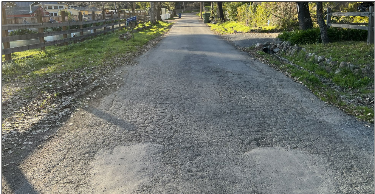
Trinity Road (Road ID: 66057) – Dunbar Road to Highway 12, Glen Ellen. Length: 0.32 Mile. Treatment: Asphalt Overlay
