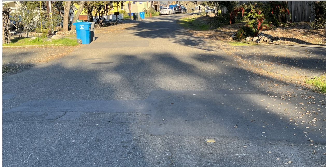
Bonnie Way (Road ID: 66074) – Dunbar Drive to Sylvia Drive, Glen Ellen. Length: 0.40 Mile. Treatment: Asphalt Overlay
