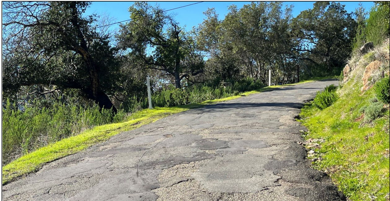
Cavedale Road (Road ID: 66032) - Highway 12 to Trinity Road, Sonoma and Glen Ellen. Length: 7.50 Miles. Treatment: Asphalt Overlay
