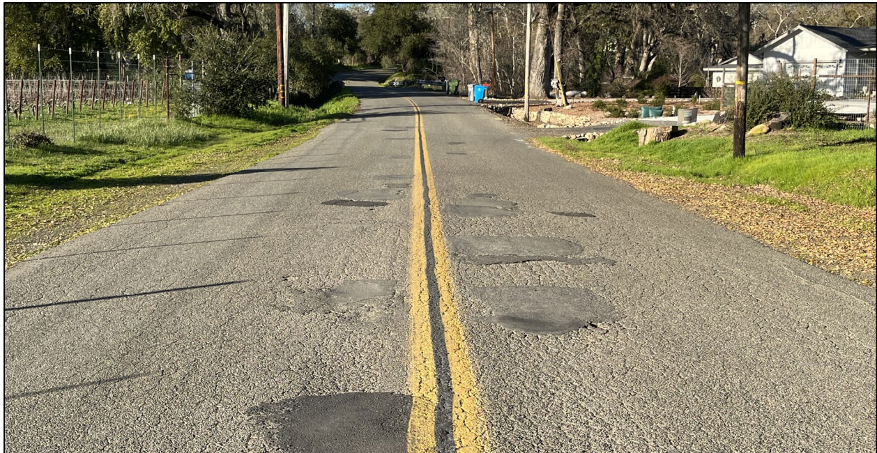
Dunbar Road (Road ID: 66056) – Arnold Drive to Highway 12, Glen Ellen. Length: 1.65 Miles. Treatment: Asphalt Overlay
