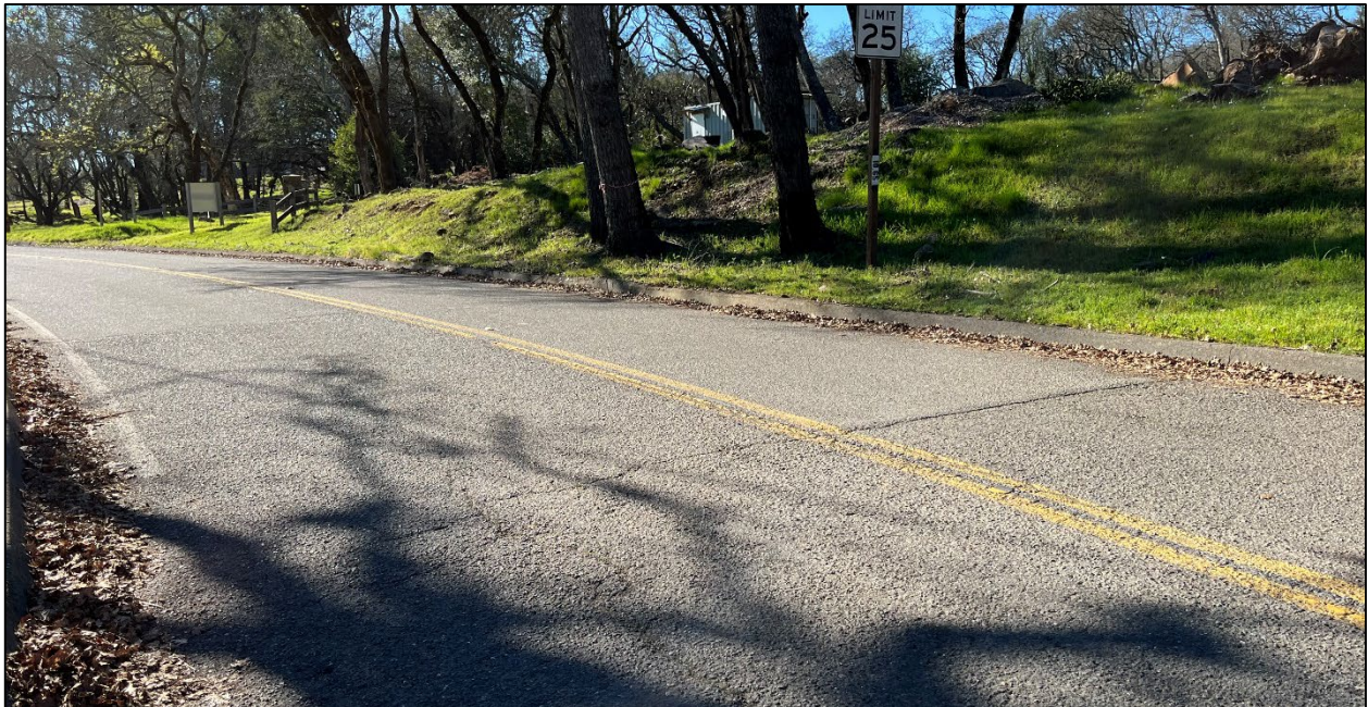
Rollo Road (Road ID: 66097) - Old Bennett Ridge Road to Bennett Ridge Road, Santa Rosa. Length: 0.66 Mile. Treatment: Asphalt Overlay
