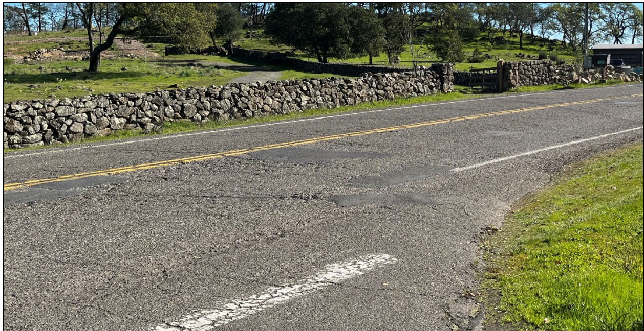
Old Bennett Ridge Road (Road ID: 66081A) - Bennett Valley Road to End of County Maintained Road, Santa Rosa. Length: 0.70 Mile. Treatment: Asphalt Overlay
