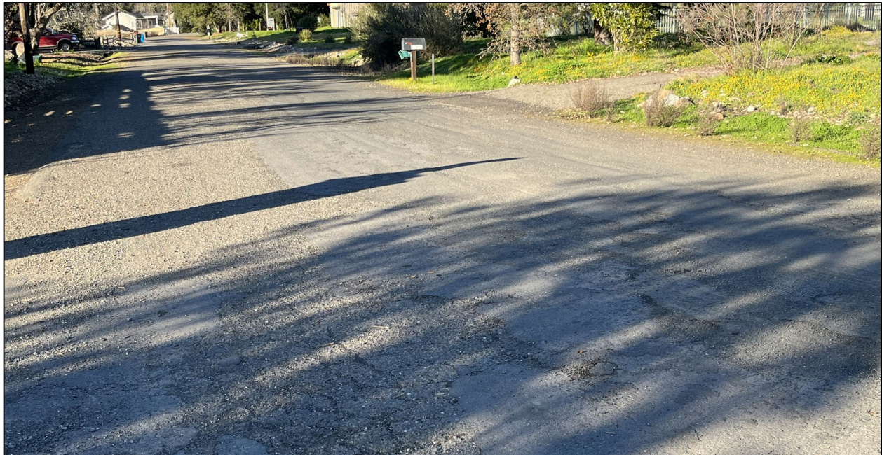
Adine Court (Road ID: 66076) – Sylvia Drive to Cul De Sac, Glen Ellen. Length: 0.15 Mile. Treatment: Asphalt Overlay
