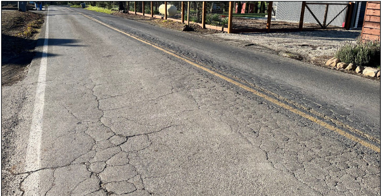
Wallace Road (Road ID: 77067) - City of Santa Rosa Limits to End of County Maintained Road, Santa Rosa. Length: 1.55 Miles. Treatment: Asphalt Overlay
