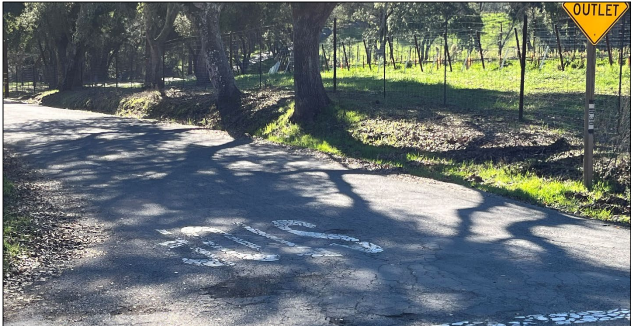
Keiser Road (Road ID: 66062) - End County Maintained Road to Lawndale Road, Kenwood. Length: 0.31 Mile. Treatment: Asphalt Overlay
