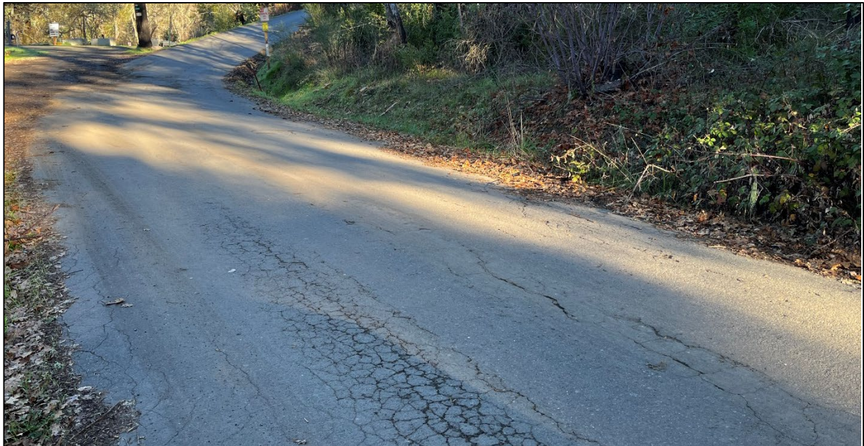
Alpine Road (Road ID: 87001) - Calistoga Road to End of County Maintained Road, Santa Rosa. Length: 0.86 Mile. Treatment: Asphalt Overlay
