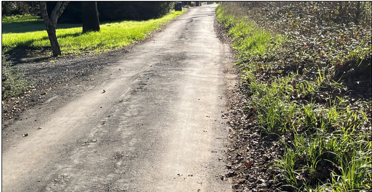
Mervin Avenue (Road ID: 76017) - End of County Maintained Road to Warm Springs Road, Kenwood. Length: 0.25 Mile. Treatment: Asphalt Overlay
