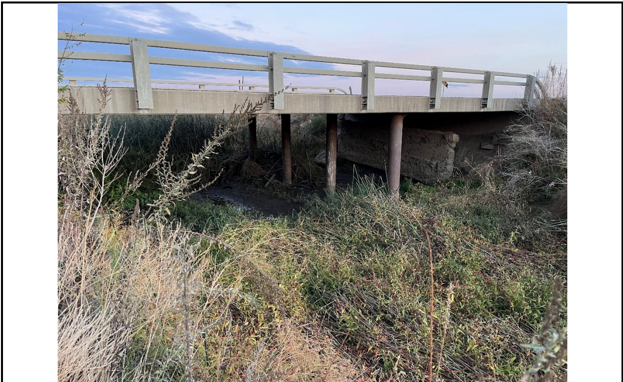
Photo 12. View of concrete bridge at S. Gurr Road crossing of Duck Slough (drainage crossing ND-7).
