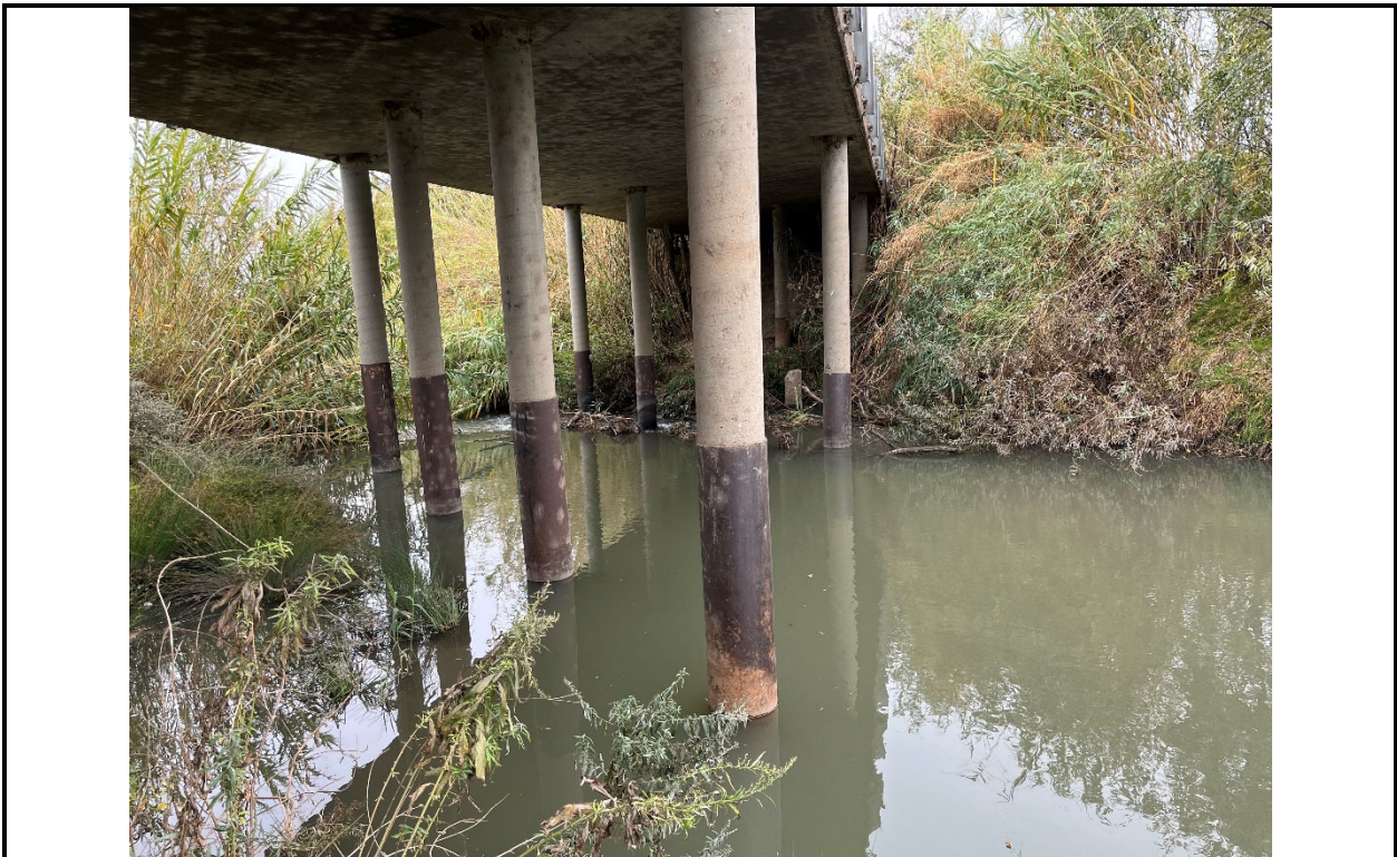
Photo 2. View of the concrete bridge at the Black Rascal Creek crossing location (drainage crossing ND-1).
