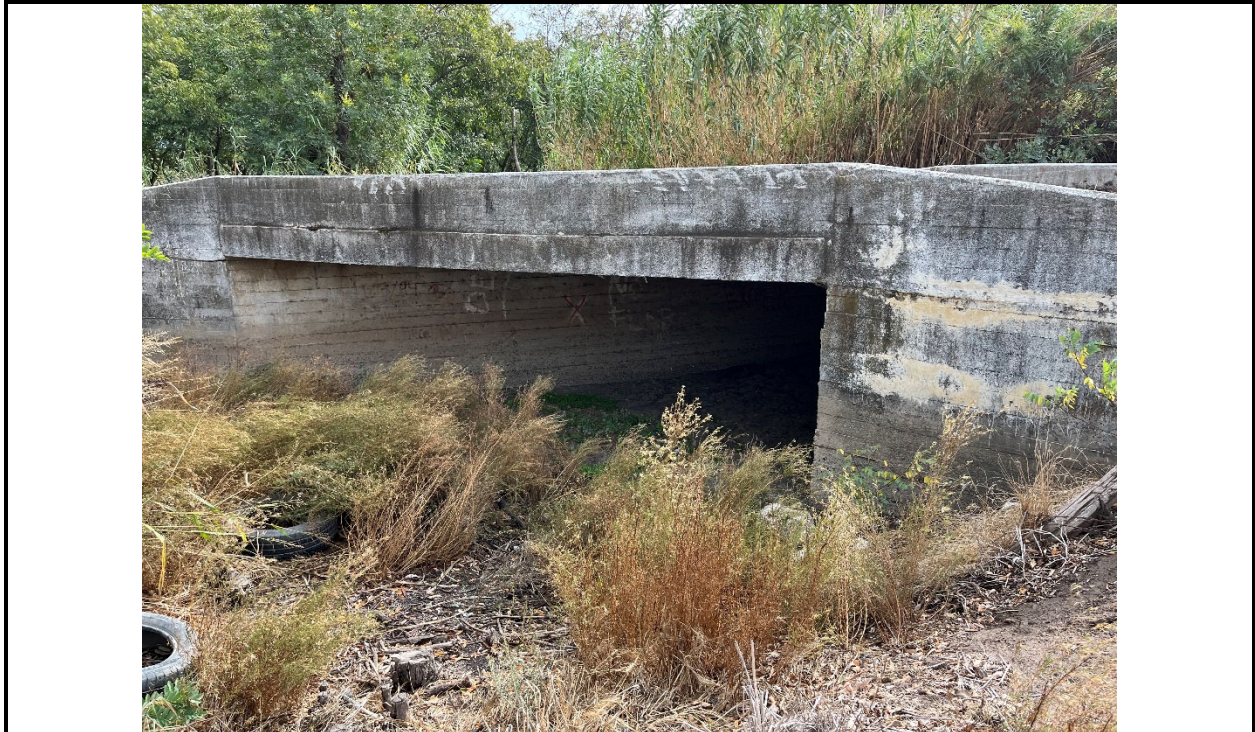
Photo 5. South view of the small concrete bridge on Oak Avenue along the proposed pipeline alignment at a natural drainage crossing (drainage crossing ND-3).
