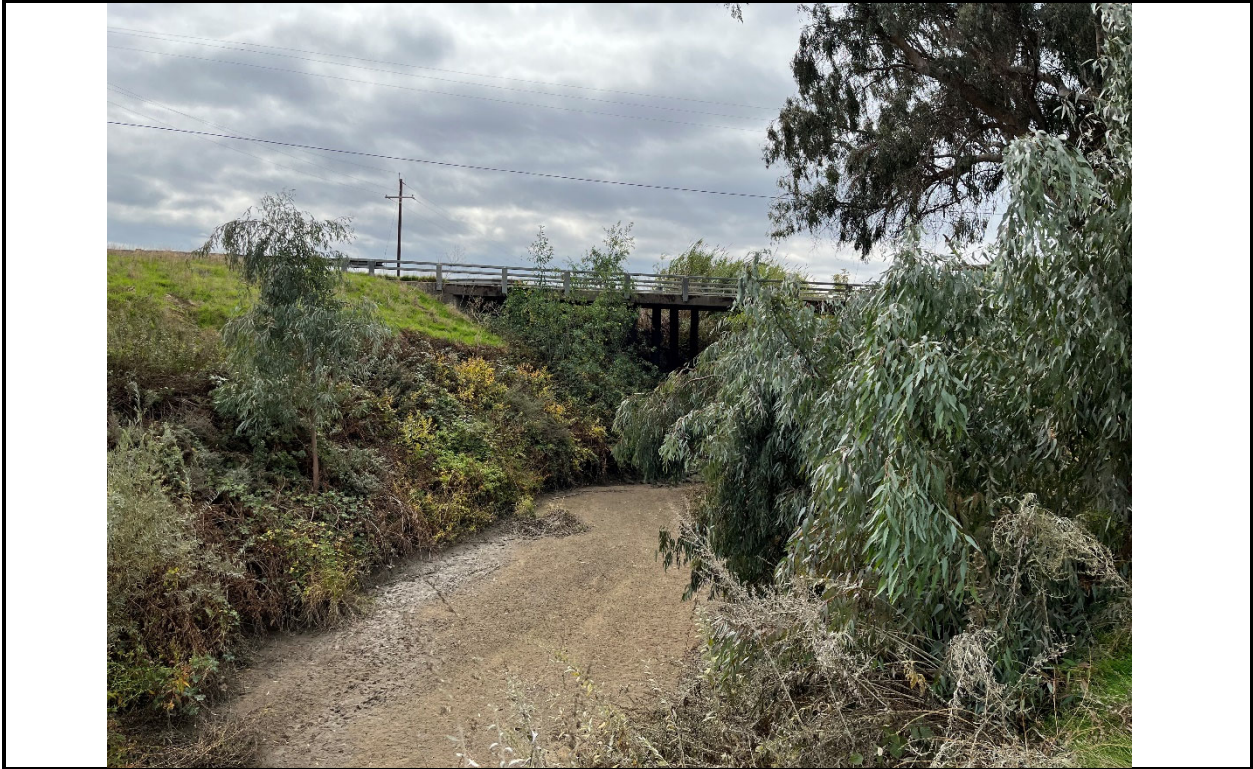
Photo 3. View of Bear Creek and the concrete bridge on Oak Avenue (drainage crossing ND-2). View south toward Oak Avenue.
