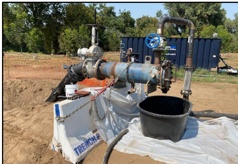
Figure 2-19. Photograph of a Sample Pig Receiver and Associated Equipment
