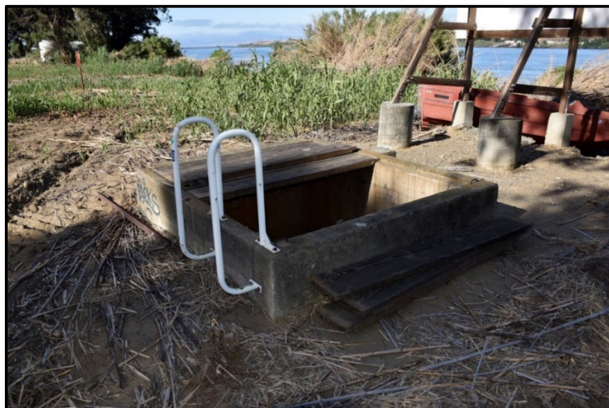
Figure 2-17. Photograph of the Concrete Valve Box Located Within the East Levee (Segment 3)
