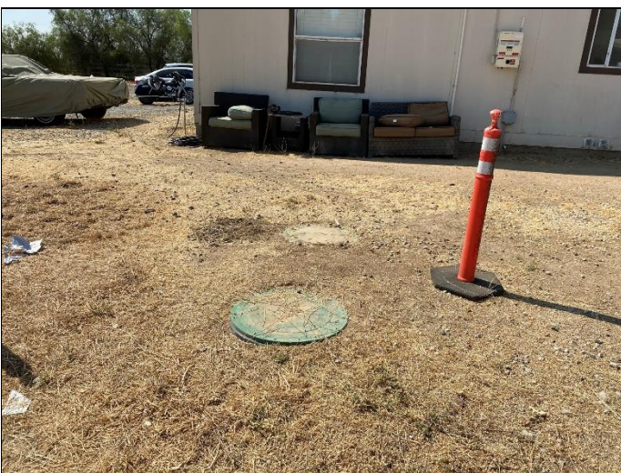
17. View of typical septic tank
