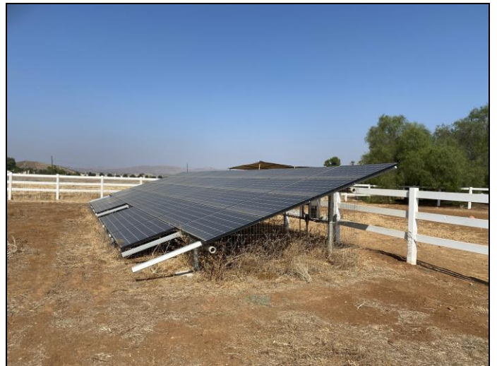
16. View of onsite solar panels
