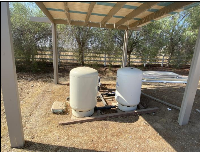
15. View of onsite water well
