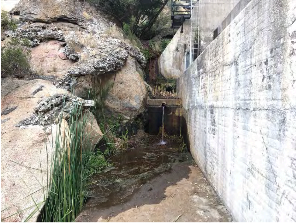
Photo 5. Barrett Dam – Seep near the bottom of the dam. Both species of treefrog often observed here. June 22, 2020.
