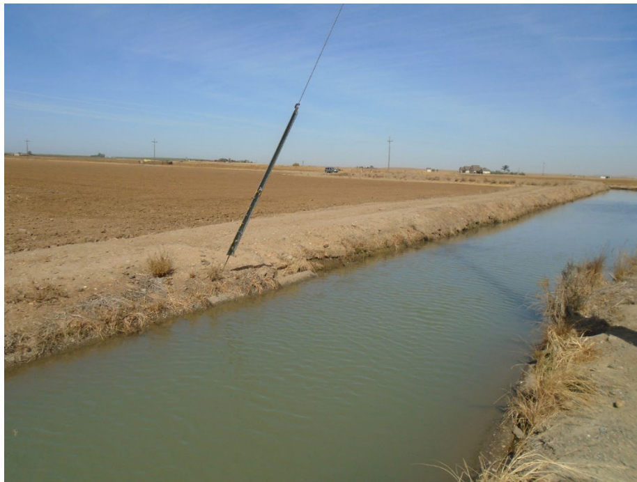
Description of Photo: Overview of heavily deteriorated segment of cement-lined canal. This segment runs roughly north-south and is approximately 685 feet long View northwest. September 20, 2021 (UTM 10N .745695 mE/ 4124712 mN).
