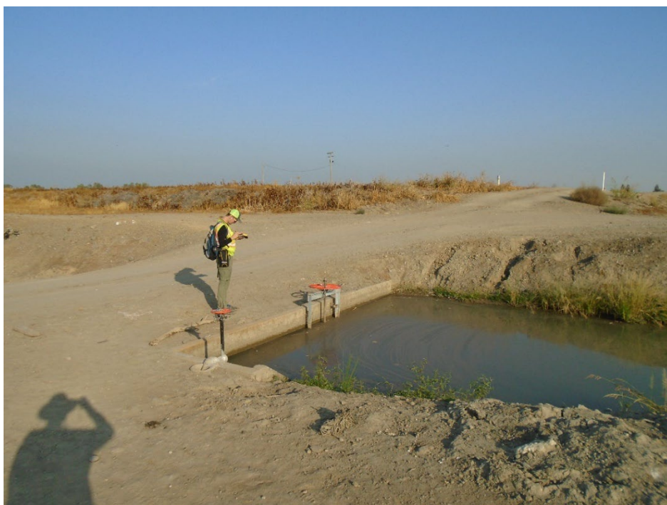
Description of Photo: Overview of F-19. View west. Sluice leads to a historic southwest-flowing canal channel. The cement portion spans the canal at this point and is approximately 22 feet long. September 22, 2021 (UTM 10N 741228 mE/ 4129329 mN).
