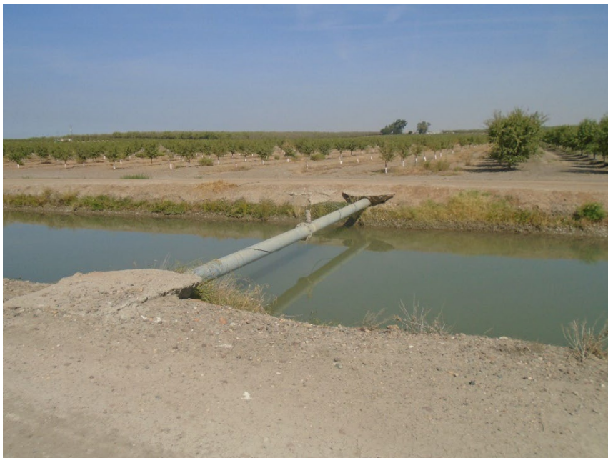
Description of Photo: Overview of F-34. View north. Metal pipe spanning the width of the Le Grand Canal. The exposed pipe is approximately 32 feet long but continues underground both north and south September 23, 2021 (UTM 10N 743083 mE/ 4125702 mN).
