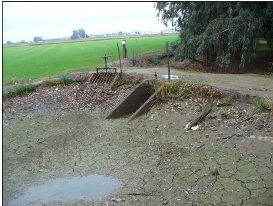
Photograph 36. East Ashe Lateral near Trinidad Road showing concrete and metal control gates at point EA6, camera facing southeast. 12/12/06
