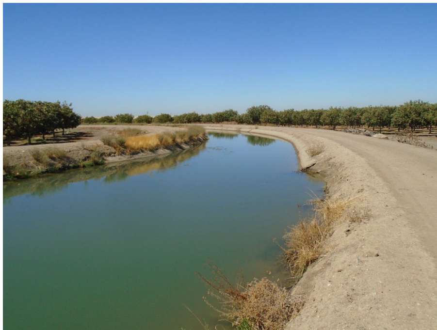
Description of Photo: Transition from earthen to cement-lined canal segment This segment is approximately 915 feet long and runs roughly northwest-southeast. View northwest. September 20, 2021 (10N 739164 mE/ 4133268 mN).
