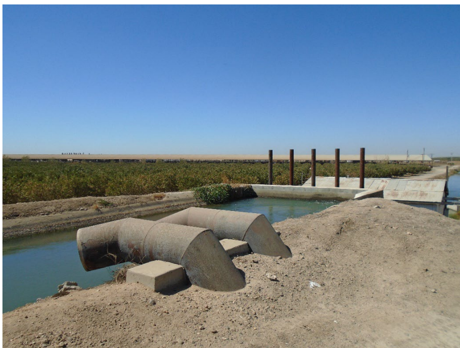
Description of Photo: F-05, cement-lined inlet and associated ferrous pipes. The top of F-06 pump house is also pictured. View north. September 20, 2021 (UTM 10N .738911 mE/ 4133255 mN)
