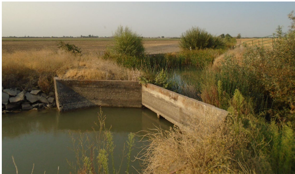
Description of Photo: Detail of F-11, a cement dam/inlet and drop. View south. September 21, 2021 (UTM 10N 740794 mE, 4132186 mN).
