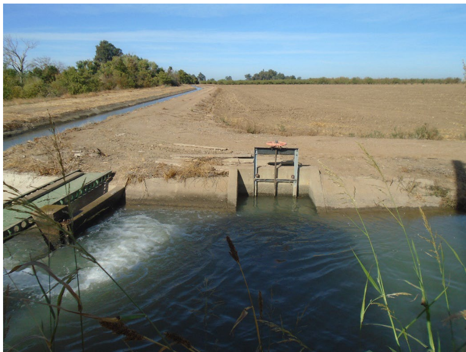
Description of Photo: Overview of F-44. View west. A tag on the sluice reads "015054 R 24 5 0 401U." September 29, 2021 (UTM 10N 745687 mE, 4124698 mN).
