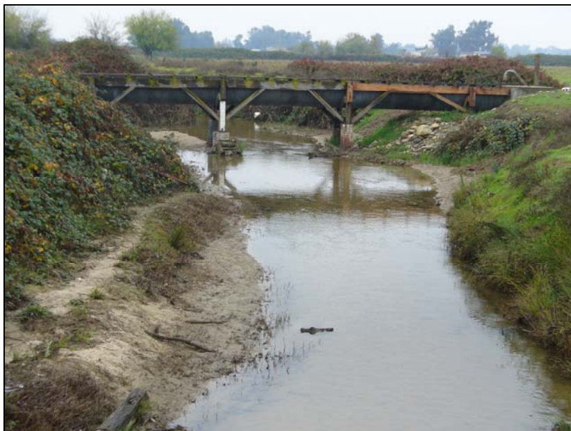
Photograph 32. Main Ashe Lateral Flume over Canal Creek at point MA2, camera facing south. 12/12/06.
