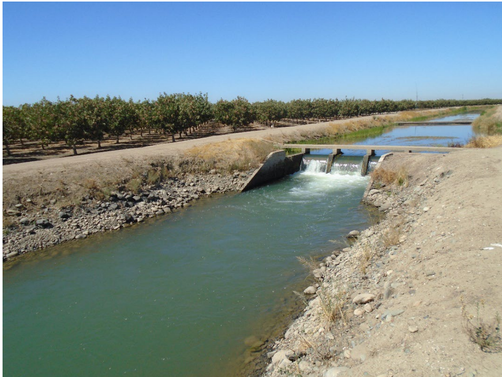
Description of Photo: F-02, concrete drop, rip-rap lining the canal. View northwest. September 20, 2021 (UTM 10N 739420 mE/ 4133019 mN).
