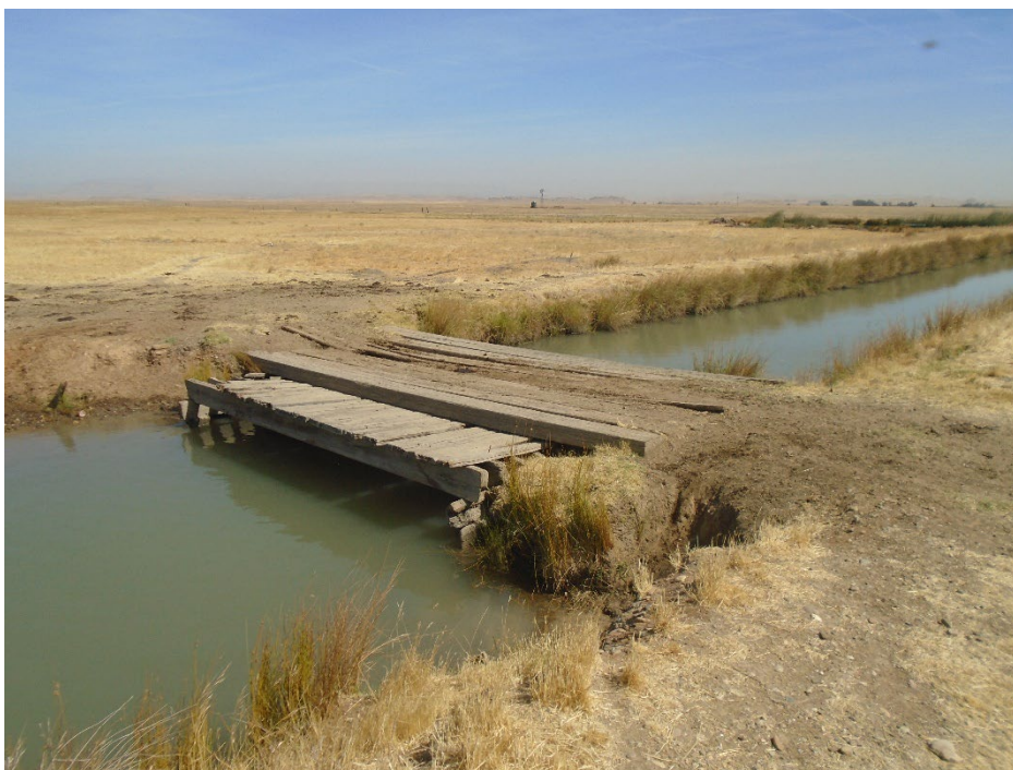
Description of Photo: F-48 overview. View northwest. Dilapidated wooden bridge spanning the Le Grand Canal. September 29, 2021(UTM 10N 745150 mE/ 4125592 mN).
