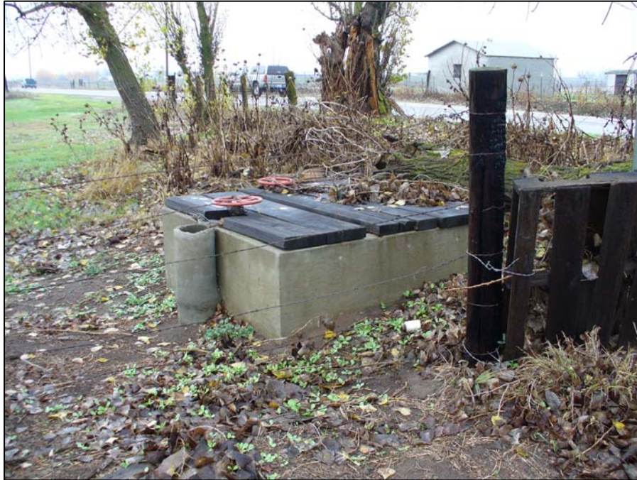
Photograph 43. Control Box at point HN2, camera facing northwest. 12/12/06.
