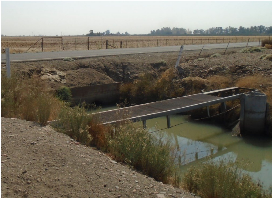
Description of Photo: Overview of F-36, west side of S. Cunningham Rd. Concrete culvert underneath S. Cunningham Rd. View southeast. September 23, 2021 (West of S. Cunningham Rd.: 7UTM 10N 43675 mE/ 4125956 mN and East of S. Cunningham Rd.: UTM 10N 743690 mE/ 4125956 mN.
