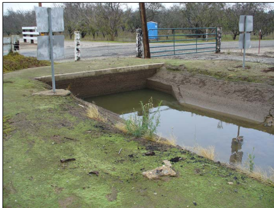
Photograph 46. Culvert under Elliot Avenue at point BH1, Buhach Lateral, camera facing northeast. 12/12/06.
