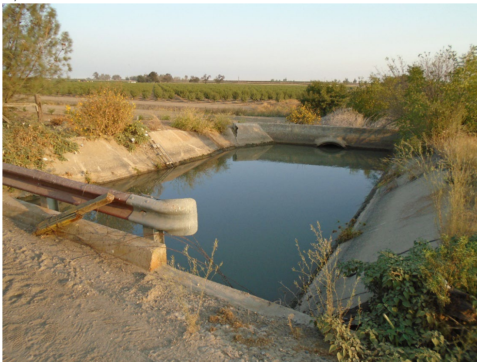
Description of Photo: F-13, cement inlet at Mission Avenue. View north. September 22, 2021 (UTM 10N . 741382 mE/ 4128635 mN).
