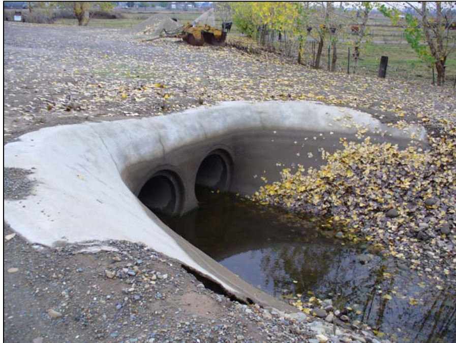
Photograph 37. Meadowbrook Lateral siphon pipes at point MB1, camera facing east. 12/12/06.
