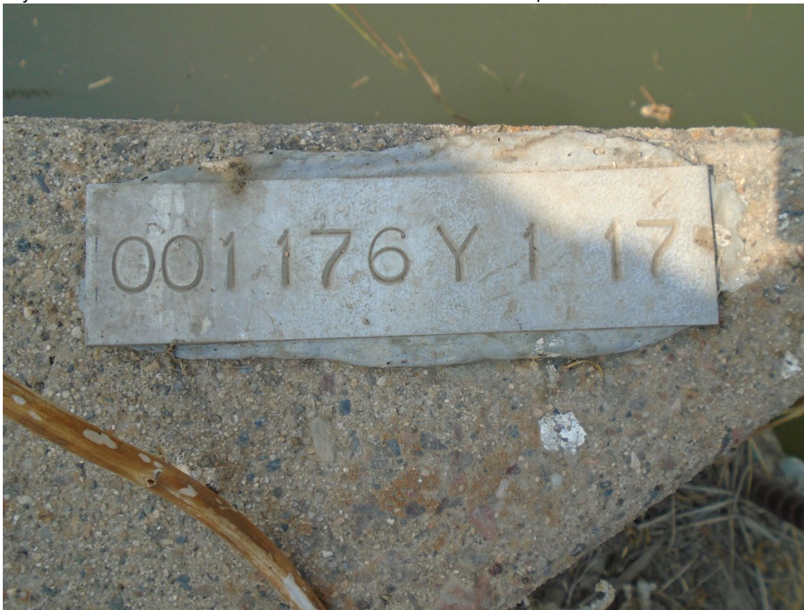
Detail photo of the metal tag observed on the cement footing.
