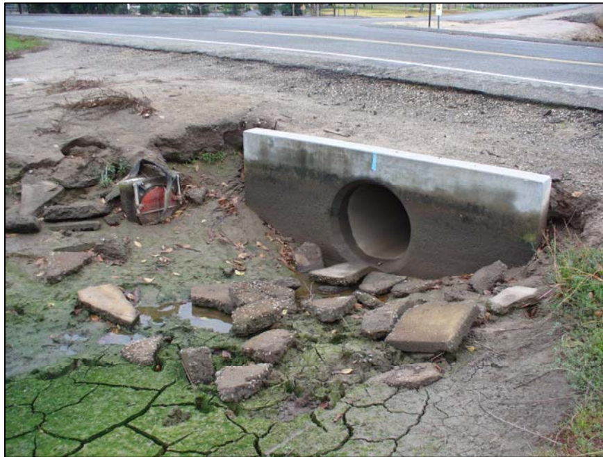
Photograph 35. Main Ashe Lateral at SP Avenue showing concrete culvert passing under SP Avenue at point MA4, camera facing southeast. 12/12/06.
