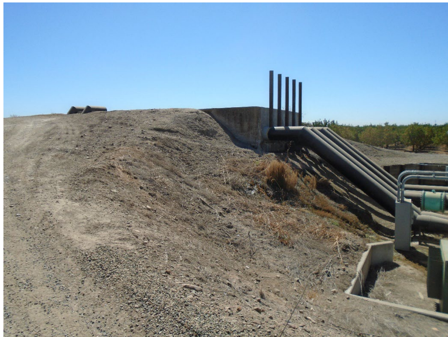
Description of Photo: North elevation of F-05 with ferrous pipes connected to the pump house (F-06). View west. September 20, 2021 (UTM 10N 738895 mE/ 4133262 mN).
