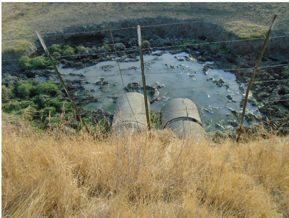
Description of Photo: F-10, cement culvert pipes, on the eastern side of the Le Grand Canal. View east. September 21, 2021 (UTM 10N 741096 mE/ 4131632 mN).
