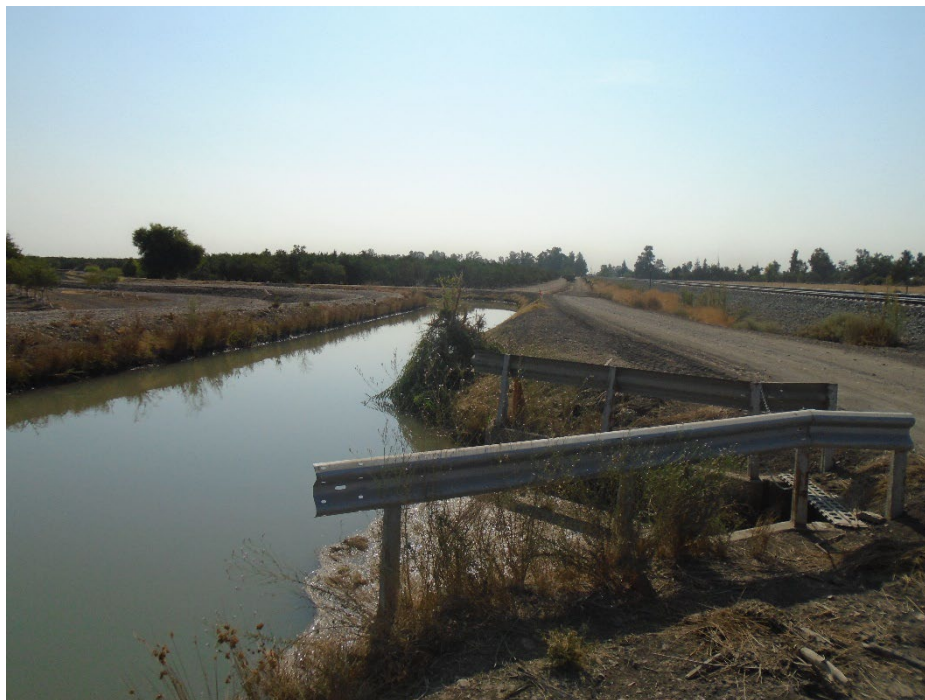
Description of Photo: View of F-32 from the northwestern corner. View southeast. Cement inlet leads to southwest flowing canal channel underneath the Santa Fe Railroad. A tag on the cement foundation reads "114059 C 1 49." September 23, 2021 (UTM 10N 742545 mE/ 4125534 mN).
