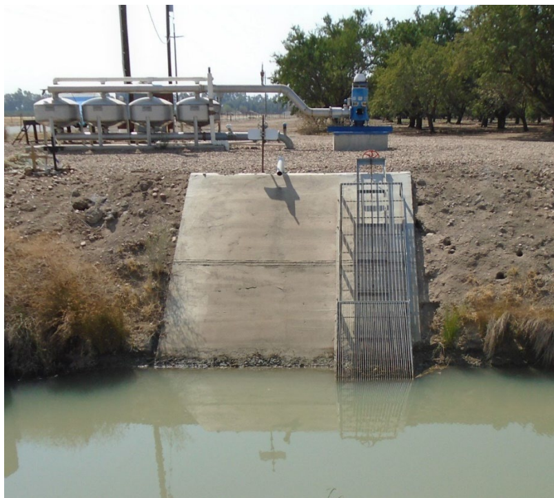
Description of Photo: F-35 overview. View south. Cement and metal sluice and associated machinery to the south. September 23, 2021 (UTM 10N Sluice:743661 mE, 4125950 mN and Machinery: UTM 10N 743667 mE, 4125941 mN).
