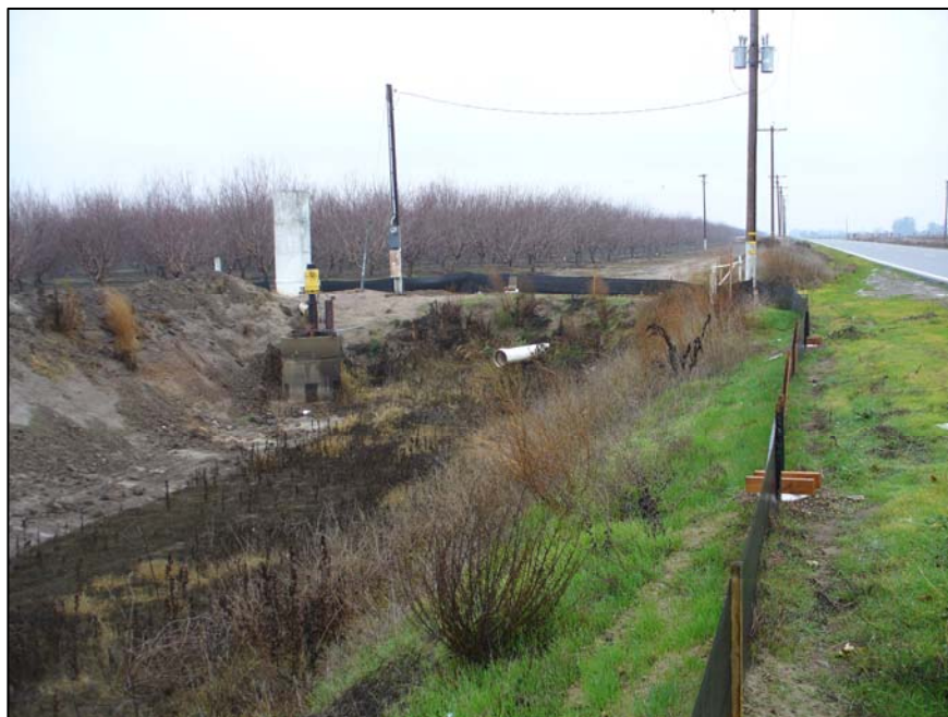
Photograph 42. Pump and vertical pipe near Henderson Lateral point HN1, camera facing northeast. 12/12/06.
