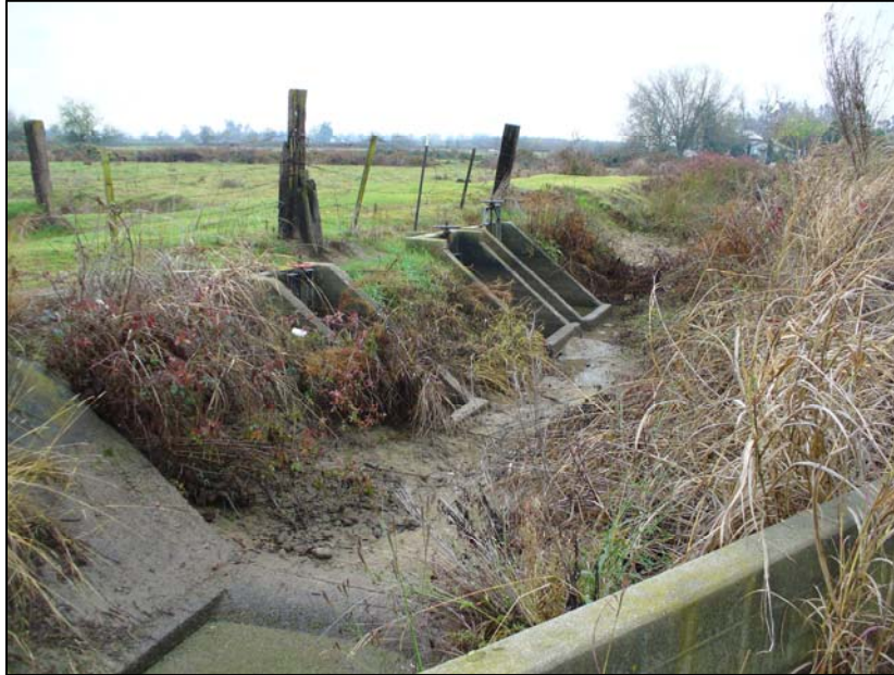
Photograph 31. Control gates on Main Ashe Lateral at point MA2, camera facing south. 12/12/06.
