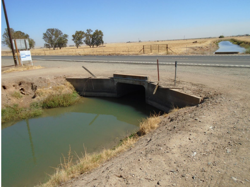
Overview of canal underneath LG-02. The canal is associated with site P-24-000608 (the Le Grand Canal). View southeast
