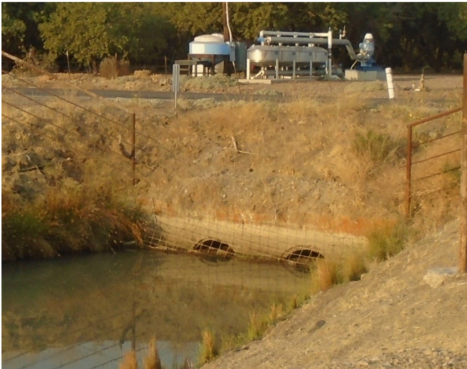
Description: Overview of F-36 on the east side of S. Cunningham Rd. September 24, 2021.
