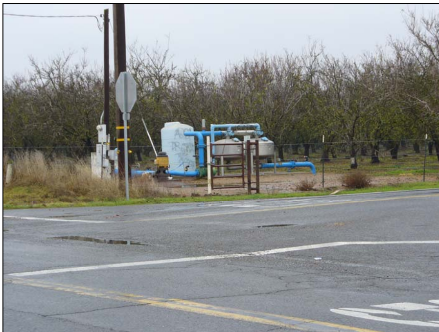
Photograph 44. Pump at point HN2, camera facing northeast. 12/12/06.
