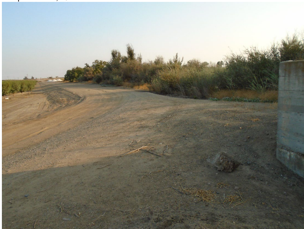
Description of Photo: Northern end of F-14 (on right) as the Le Grand Canal flume dives under the pictured access road. View northeast. September 22, 2021.
