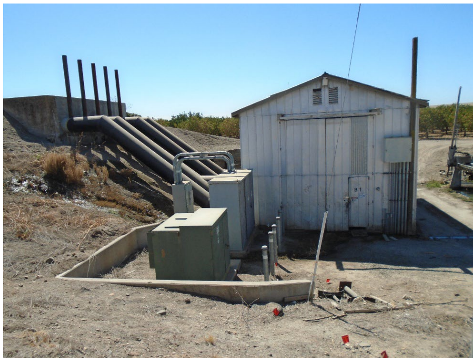
Description of Photo: East elevation of pumphouse (F-06), a pump. Ferrous pipes connect the pump house to F-05, a cement-lined inlet. View west. September 20, 2021 (UTM 10N 738895 mE/ 4133262 mN).
