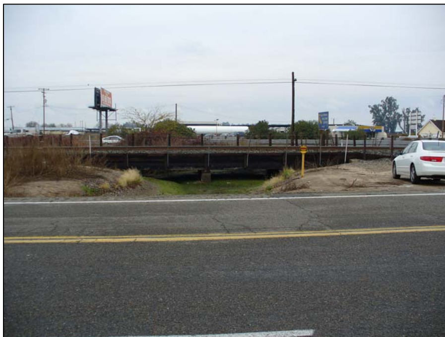
Photograph 34. Main Ashe Lateral at SP Avenue showing the canal passing under the UPRR at point MA4, camera facing north. 12/12/06.
