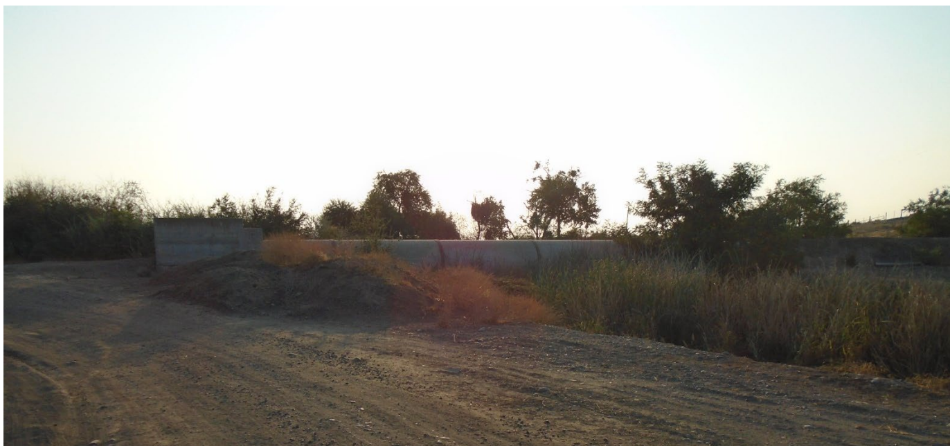
Description of Photo: Overview of F-14, a cement flume that allows water from the Le Grand Canal to dive underground. F-13 runs northwest to southeast and is approximately 190 feet long and 7 feet wide. The Le Grand Canal flows underground along a dirt access road north of this pipe for approximately 2,000 feet. The southern portion of the pipe, a 95-foot segment that intersects with F-12, is at ground level but covered with dirt. The northern end is exposed View east. September 22, 2021 (UTM 10N 741369 mE, 4128700 mN [north recorded terminus] and UTM 10N 741382 mE, 4128644 mN [south recorded terminus]).
