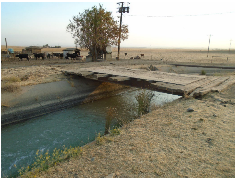
Description of Photo: F-39 overview. View northeast. Badly dilapidated wooden bridge spanning the Le Grand Canal. The bridge is approximately 23 feet long (southwest-northeast) and 12 feet wide (west-east). September 24, 2021 (UTM 10N 744246 mE/ 4126035 mN).
