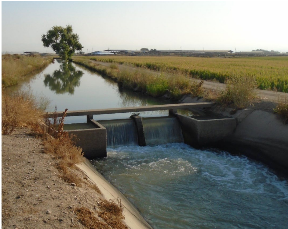
Description of Photo: F-18, cement drop. The drop spans this portion of the Le Grand Canal and is approximately 25 feet long View north. September 22, 2021 (UTM 10N 741249 mE/ 4129328 mN).
