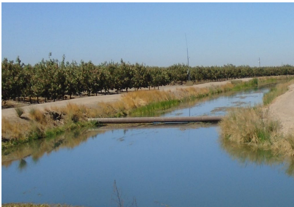
Description of Photo: F-03, ferrous pipe crossing the Le Grand Canal. View northwest. September 20, 2021 (UTM 10N 739391 mE/ 4133039 mN).
