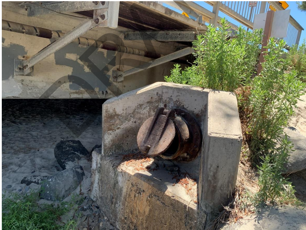
Photograph 10 - View of storm drain outfall pipe located southwest side of the bridge structure.
