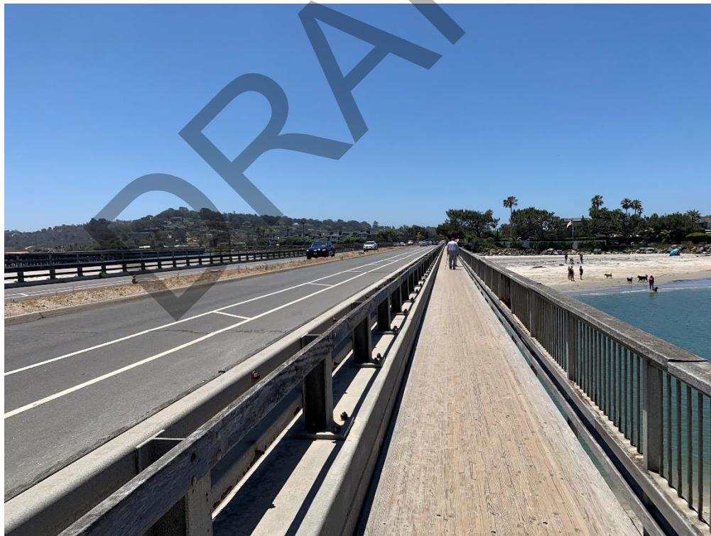
Photograph 8 - View of pedestrian walkway along the west side of bridge structure, looking south.
