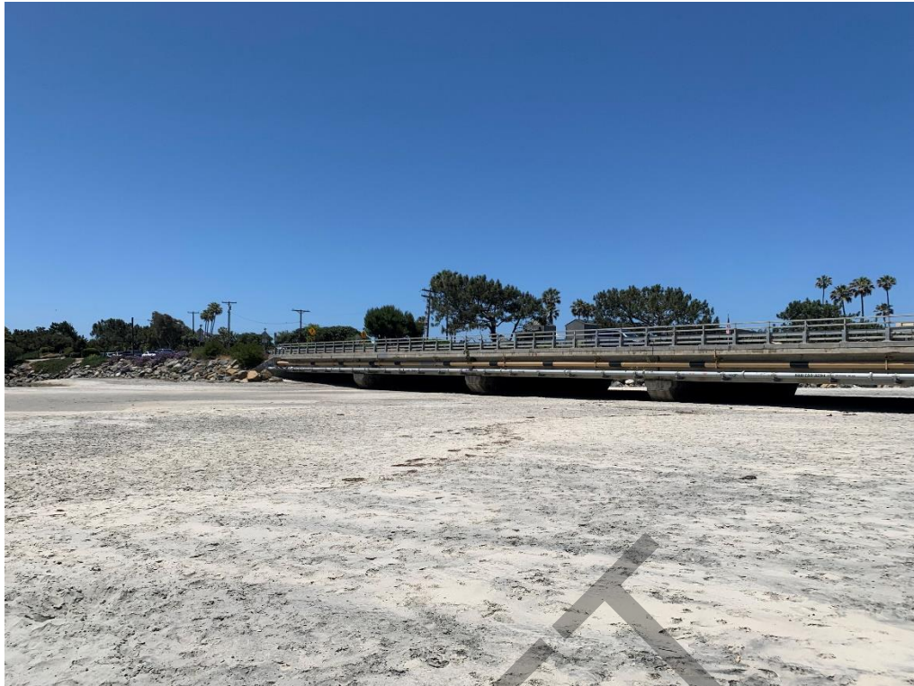
Photograph 1 - View of Camino Del Mar Bridge from east side of bridge structure, looking southwest.
