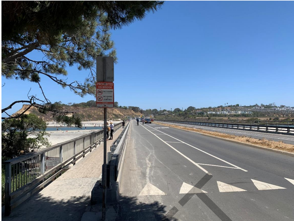
Photograph 9 - View of pedestrian walkway along the west side of bridge structure, looking north.
