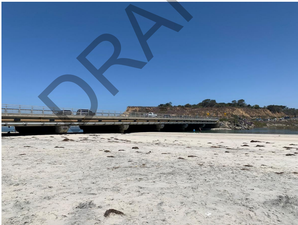
Photograph 2 - View of Camino Del Mar Bridge from east side of bridge structure, looking northwest.
