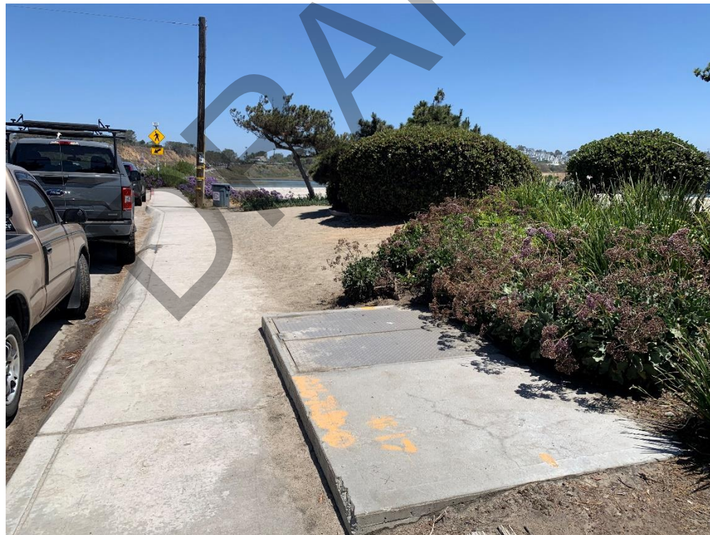
Photograph 12 - View of utility vault located east of Camino Del Mar, looking north.
