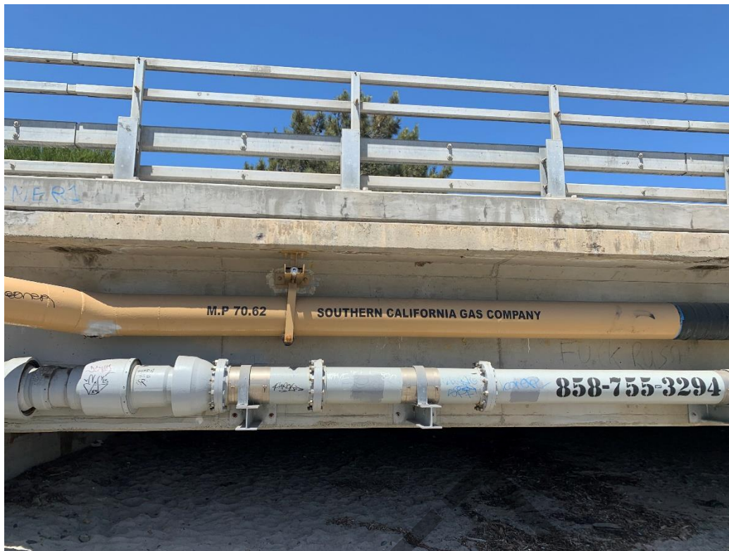
Photograph 3 - View of 12-inch natural gas pipeline and apparent City of Del Mar water line running beneath the east side of bridge structure, looking west.
