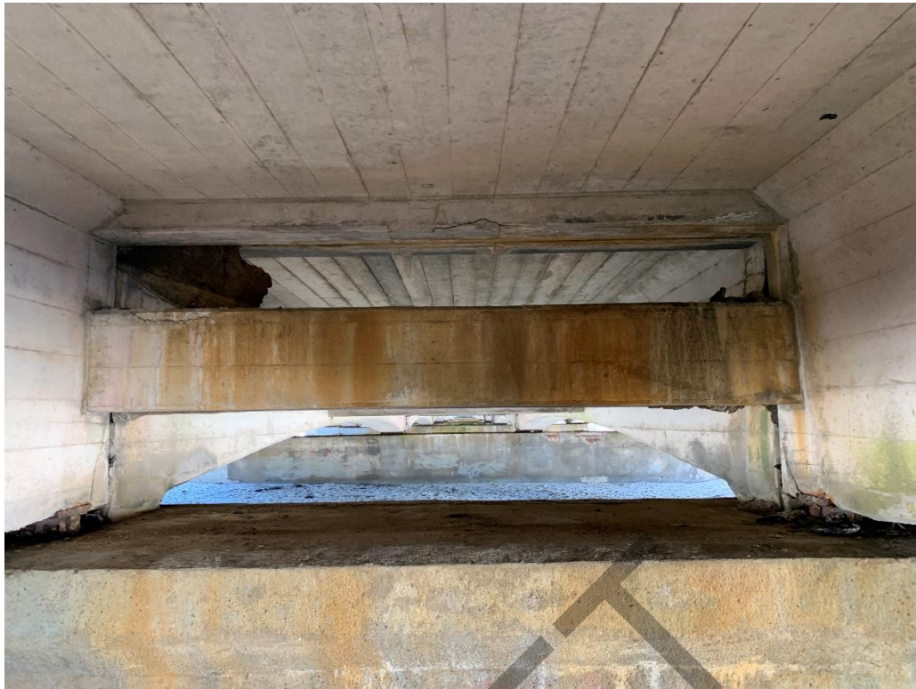
Photograph 7 - Close view of southern concrete support structures from underside of Camino Del Mar Bridge.
