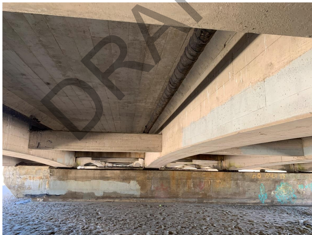
Photograph 6 - View of south bridge abutment and apparent 4-inch natural gas pipeline from underside of Camino Del Mar Bridge, looking north.
