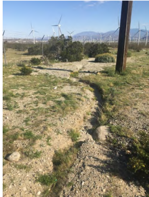
PP-6: Downstream, Southeast-Facing View of roadside ditch collecting runoff from Diablo Road along generation tie line alignment.. Near Ordinary High Water Mark Data Point (ODP)-3
