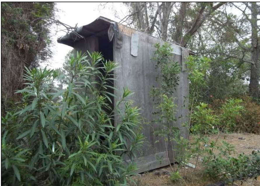
Figure 9. 1190 Island View Lane, shed, south façade (left) and east elevation (right), facing west
