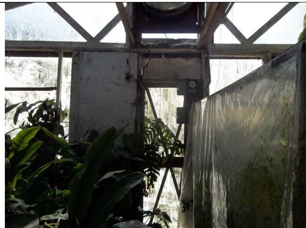
23. Interior, ventilation equipment at east elevation
