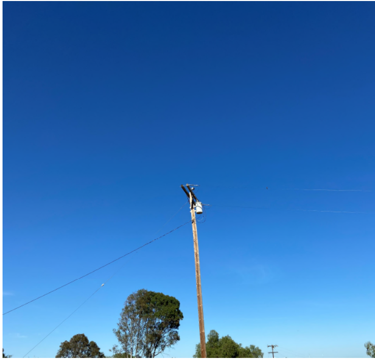
Photograph #17 Pole-mounted transformer in the central portion of the Site.
